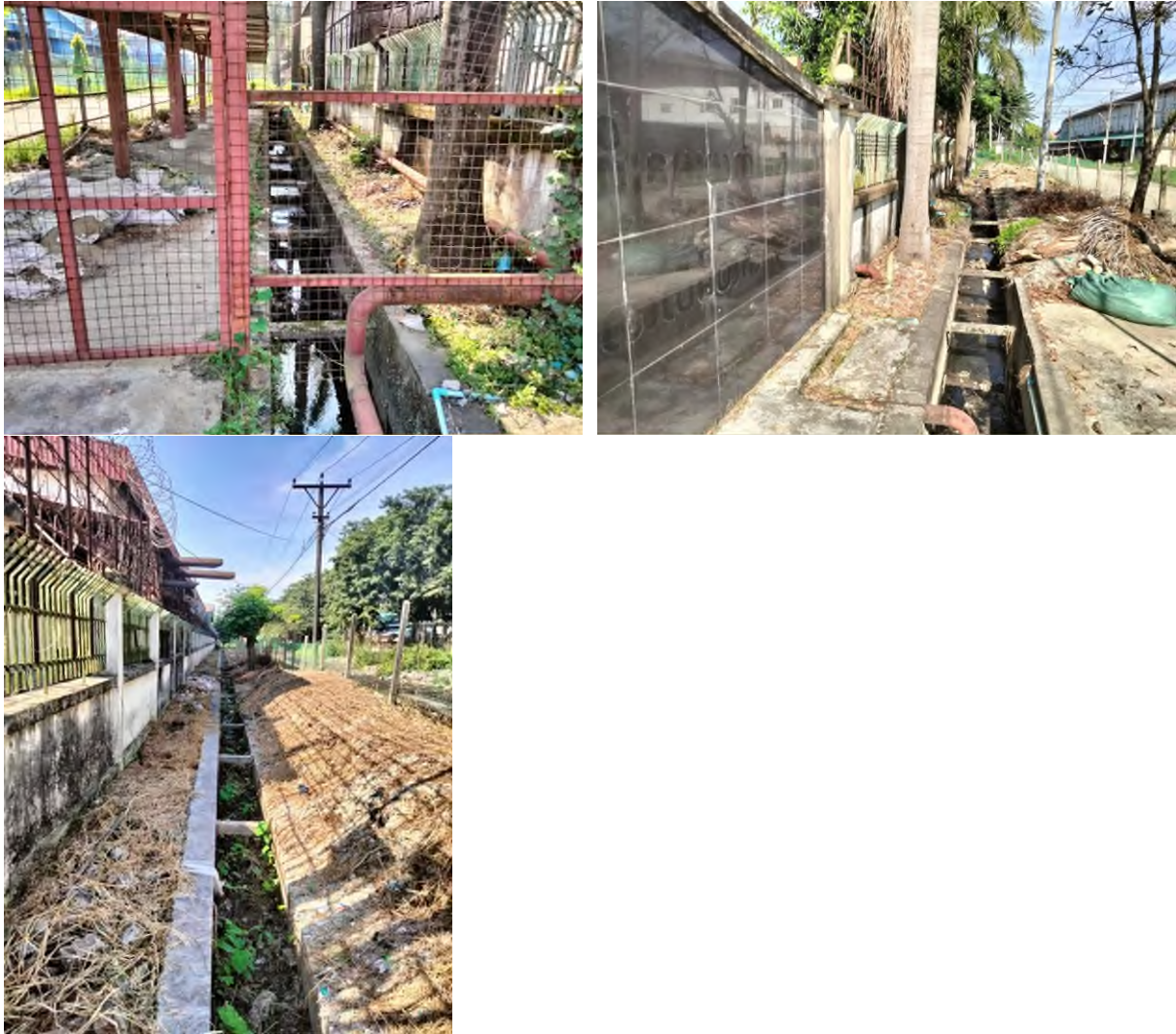
Figure 24: Drainage System at Factory
