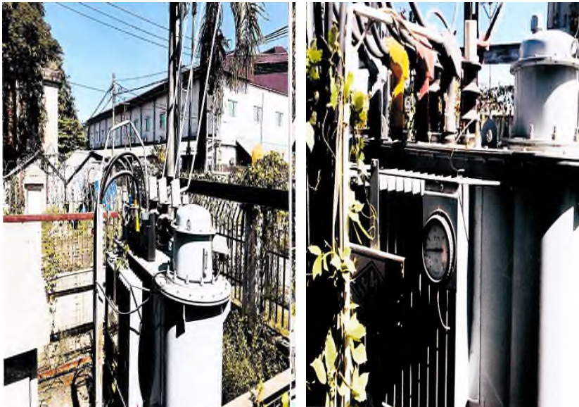
Figure 17: Own Transformer (429 KV=2)
