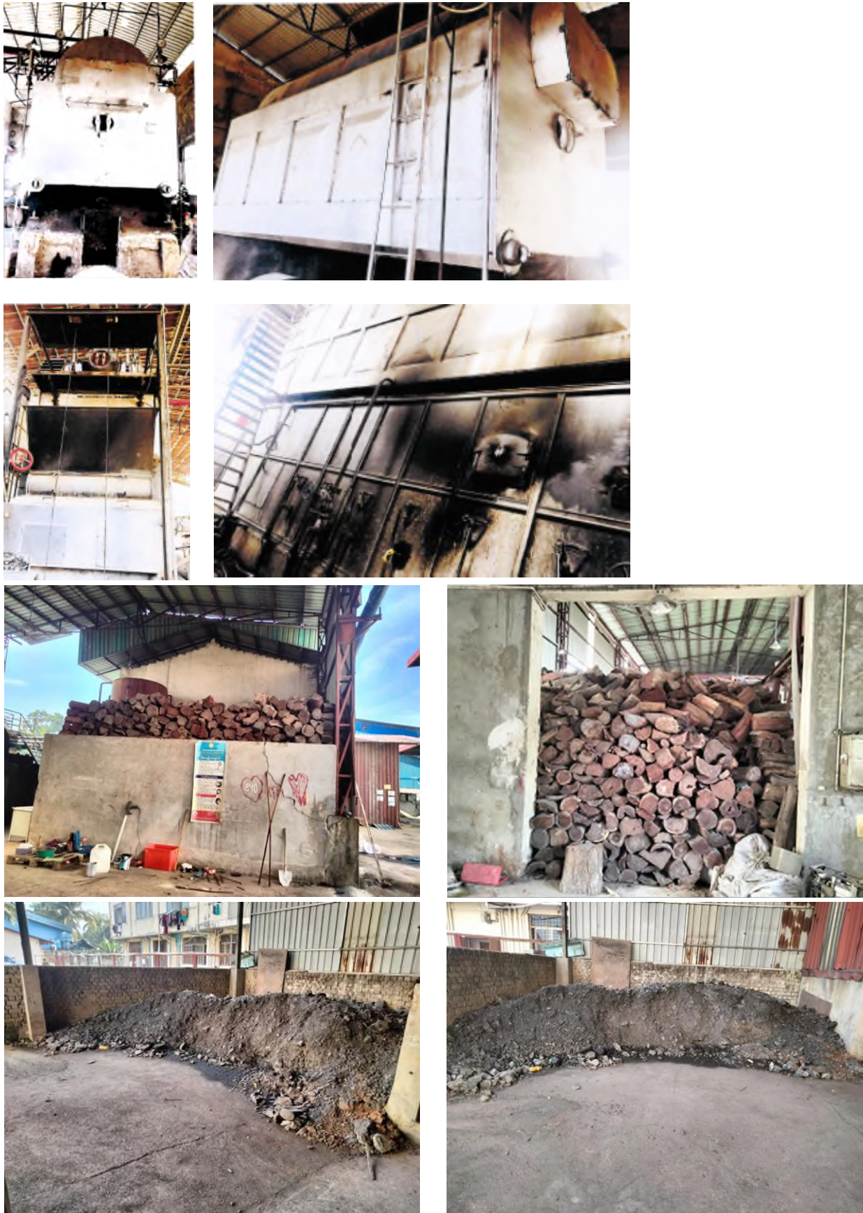
Figure 18: 4 ton & 10-ton Boilers at Jinli Factory and Coal and Firewood Storage
