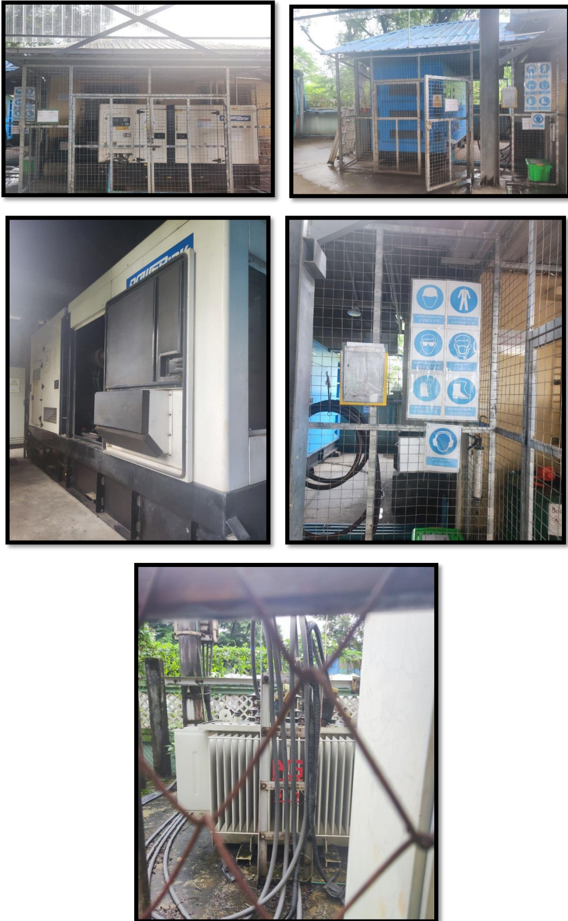
Figure 3-13 Photos of Transformer and Generator
