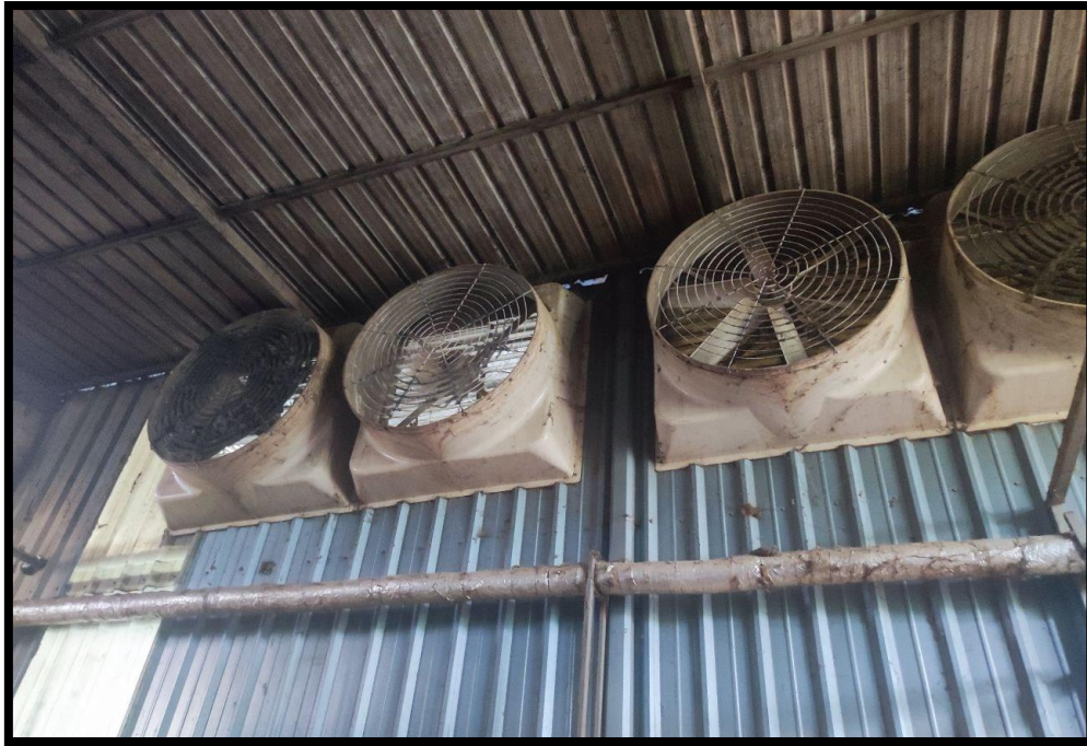
Figure 3-19 Photos of Ventilation
