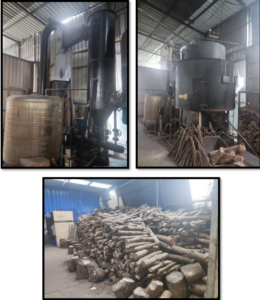
Figure 3.15 Photo of Boiler, fuel
