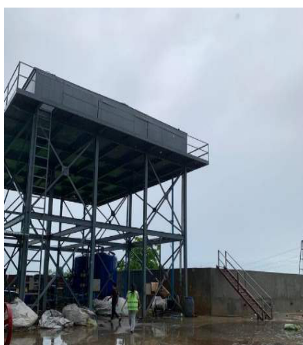
Figure 4.15- Wastewater Treatment System in Factory 2
