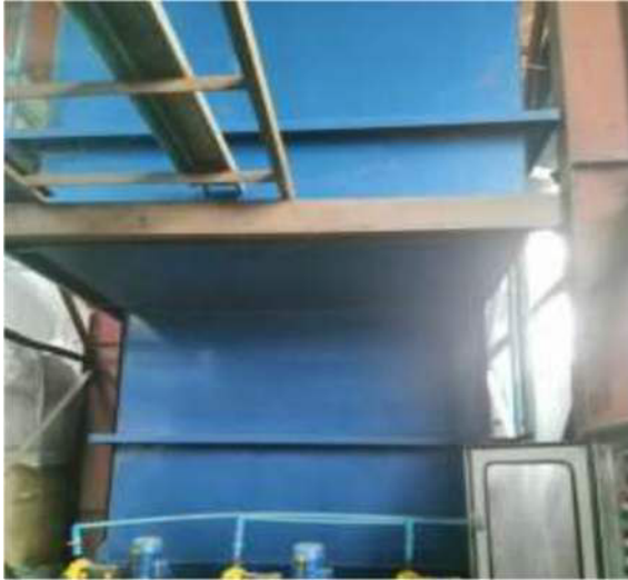
Wastewater Treatment System in Factory 1
