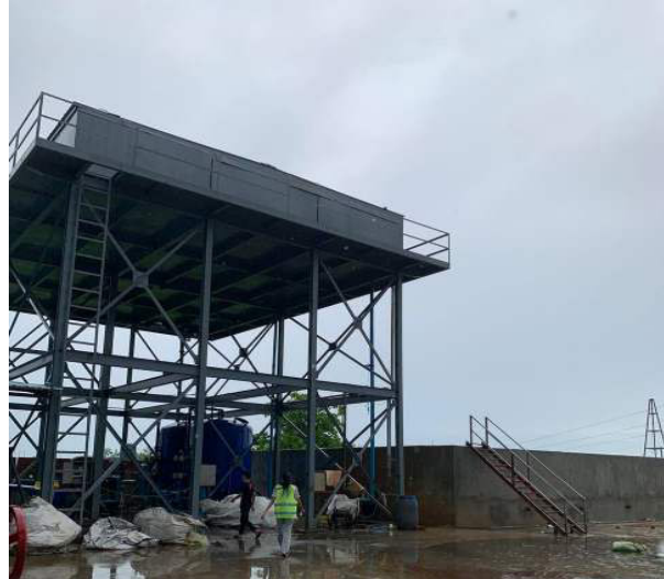
Wastewater Treatment System in Factory 2
