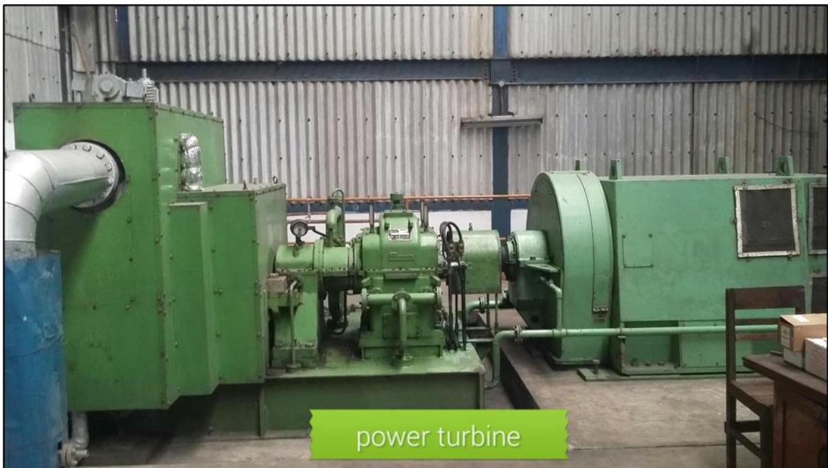
Figure 3.7: Power Turbine Generator
