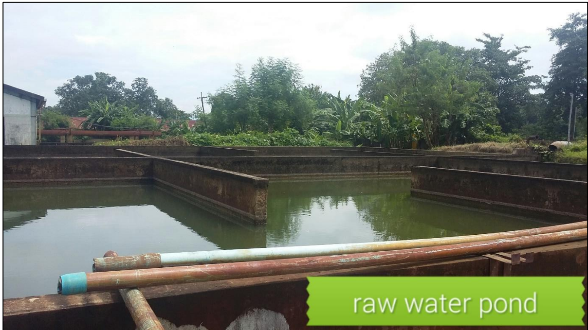
Figure 3.9: Raw Water (River water) Storage Area
