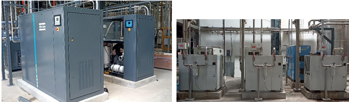
Figure 3-18 photos of air plant
