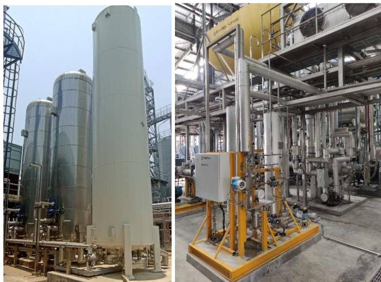
Figure 3-16 photos of CO 2 recovery plant
