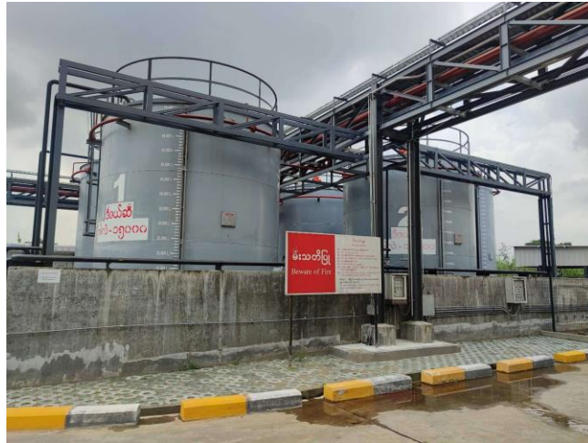
Figure 3-24 Three Diesel Tanks (Capacity - 15000 Gallons) with containment
