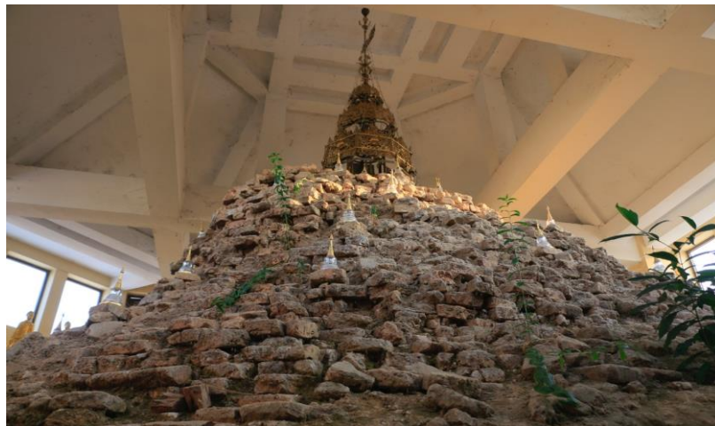
Figure 4-87 Original brick top of North Iccapunna Stupa encased by the new RC structure
