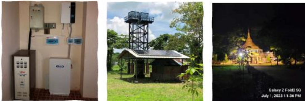
Figure 8-7 5 kW solar electric system for Amawatty Monastery
