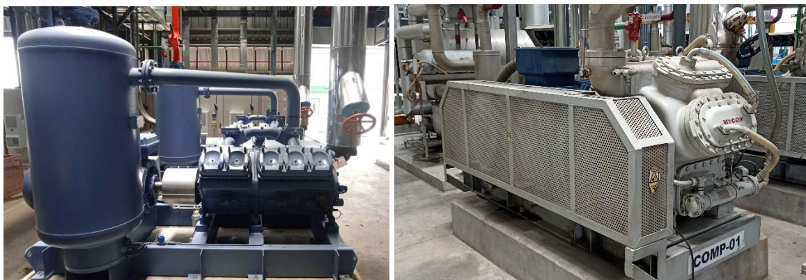
Figure 20 photos of compressors
