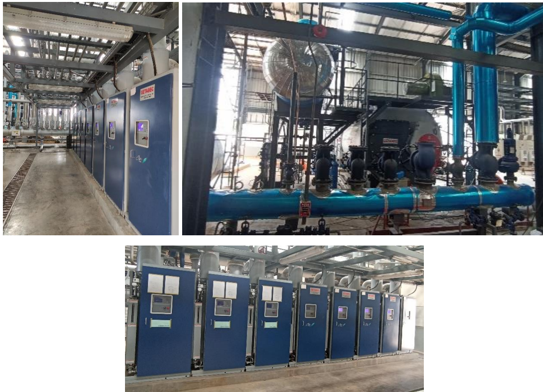
Figure 3-13 photos of boiler section
