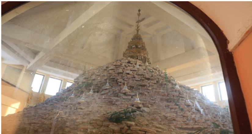
Figure 4-86 Original brick top of North Iccapunna Stupa encased by the new RC structure
