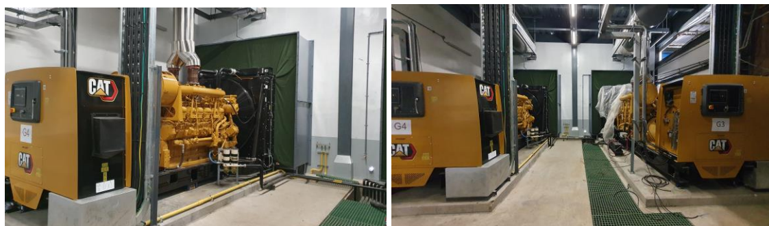
Figure 3-22 photos of generator section
