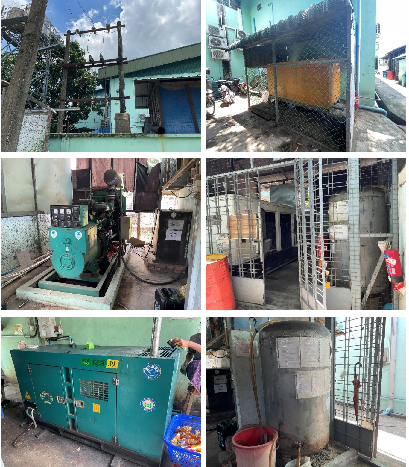
Figure 3-11 Electricity Facilities, Generator Room and Diesel Storage Area
