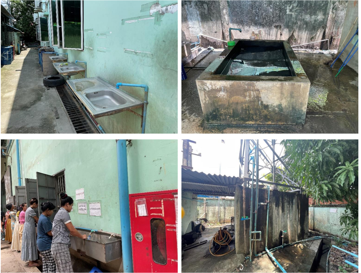
Figure 3-10 Water Storage Tank and Drinking Water Supply
