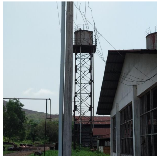
Figure 3.35 Outdoor Over Head Tanks
