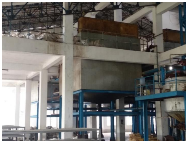
Figure 3.15 Raw Materials Tank
