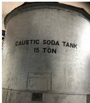
Figure 3.18 Caustic Soda Tank
