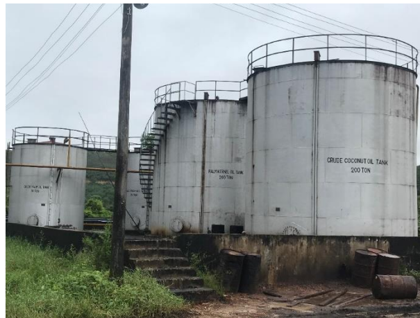
Figure 3.19 Crude Palm Oil Tank
