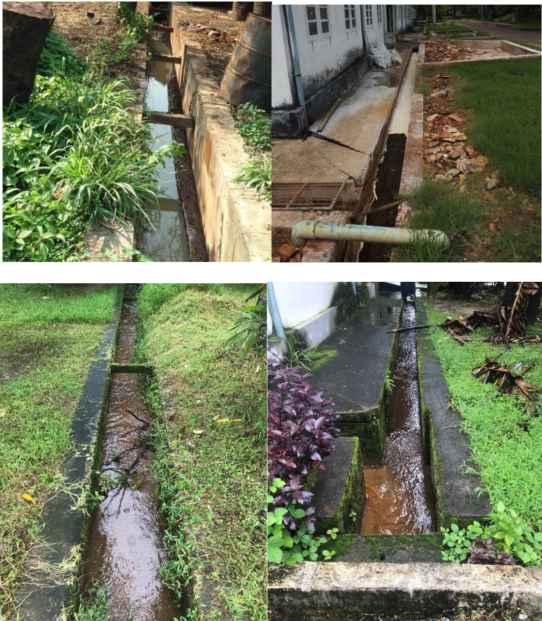
Figure 3.36 The Concrete drainage Systems within the factory areas
