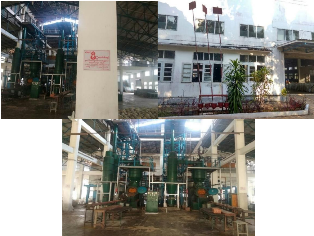
Figure 7.1 In-House Fire Fighting Equipment and Warning Signage
