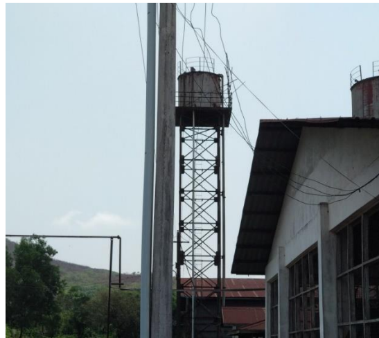
Figure 3.26 Outside Water Tank
