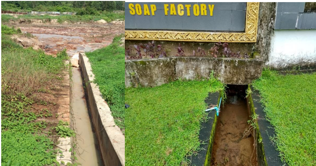
Figure 3.37 The Concrete drainage Systems outside the factory area
