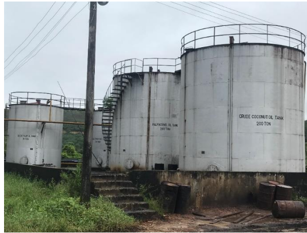
Figure 3.19 Crude Palm Oil Tank
