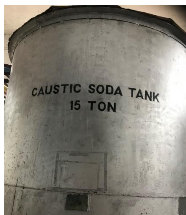
Figure 3.18 Caustic Soda Tank
