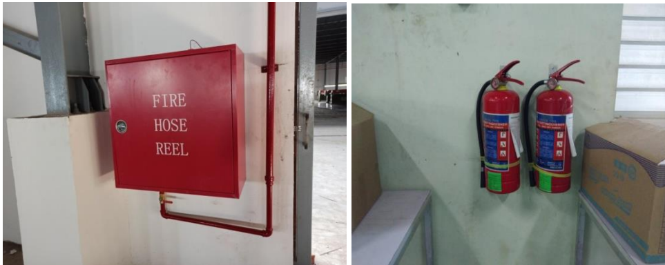
Figure 36. Fire extinguishers, fire hose cabinets and fire alarm is provided for emergency cases
