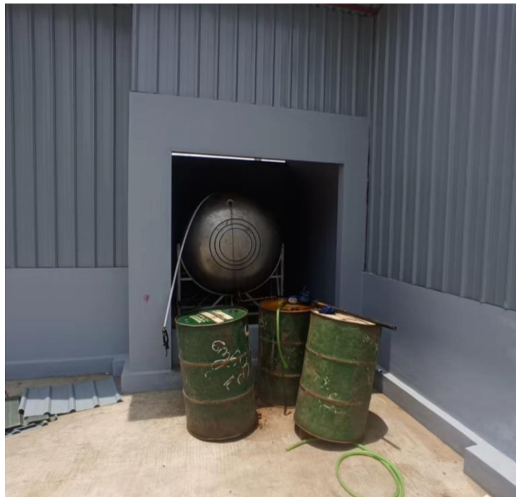
Figure 14. Diesel fuel storage with Steel Tank
