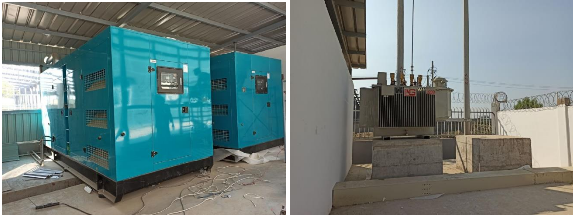
Figure 13. Generator and Electricity Transformer Storing Area
