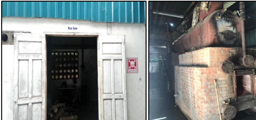
Figure 3-9 Boilers Used in Factory
