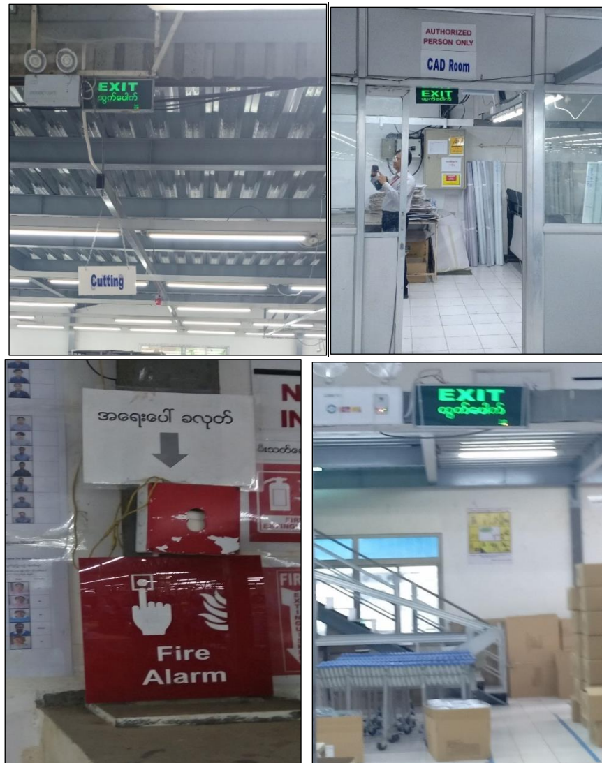
Figure 6-5 Fire Fighting Equipment and Exit Signs
