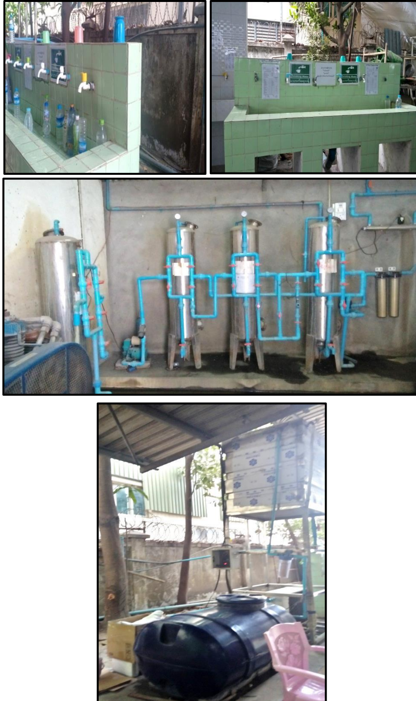
Figure 3-13 Drinking Water and Water Taps for Hand Washing
