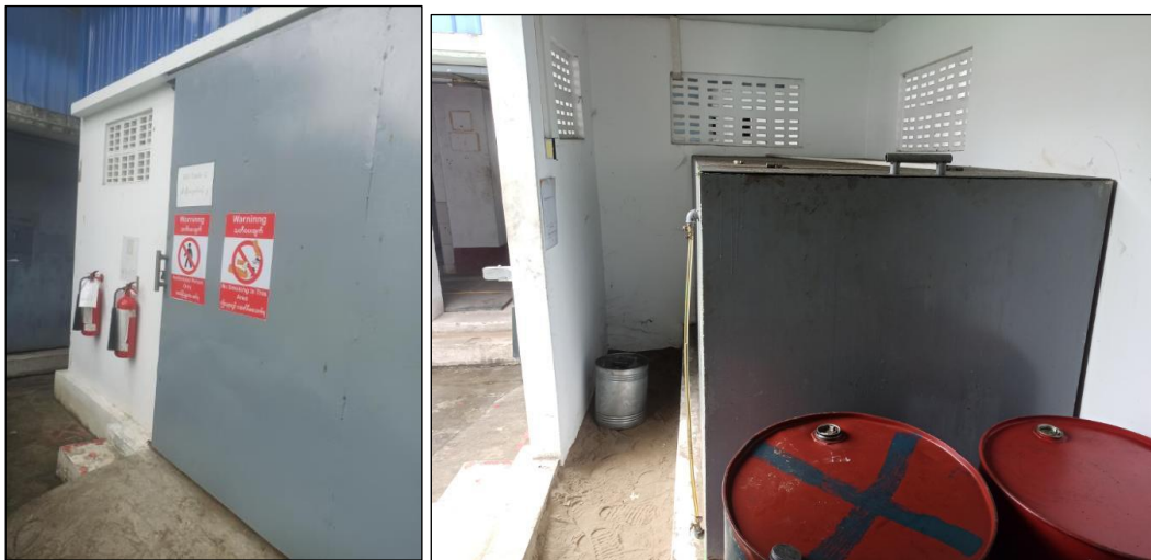
Figure 3-12 Diesel Storage Room
