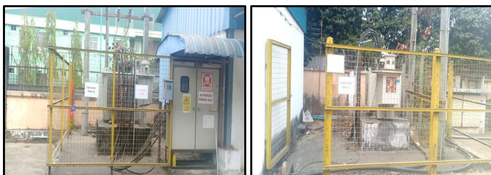
Figure 3-7 Transformer Used in Factory
