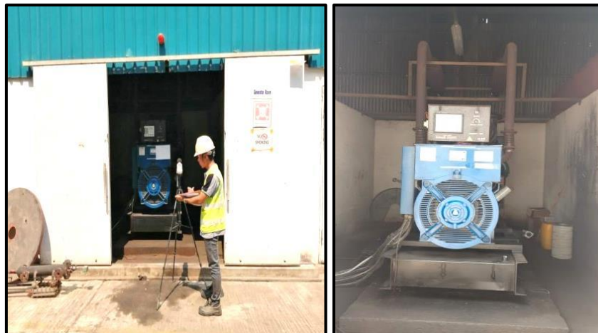
Figure 4-7 Generators Stack Emission Measuring
