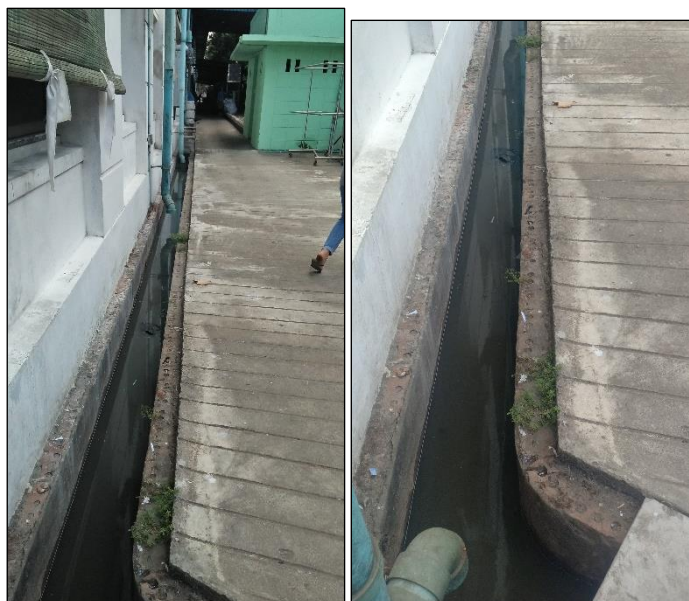
Figure 3-35 Photos of Drainage
