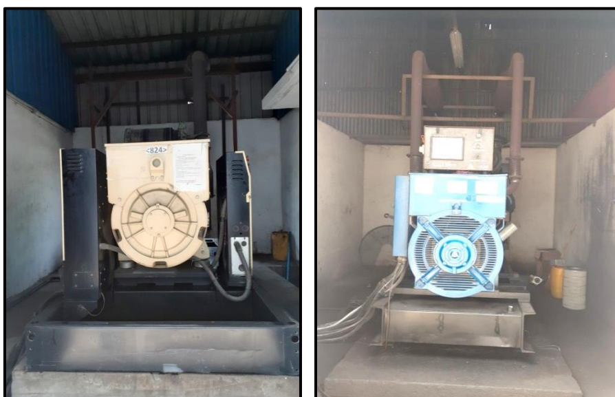
Figure 3-8 Generator Used in Factory
