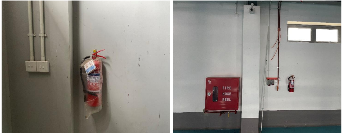
Figure 3-19 Firefighting installation photo
