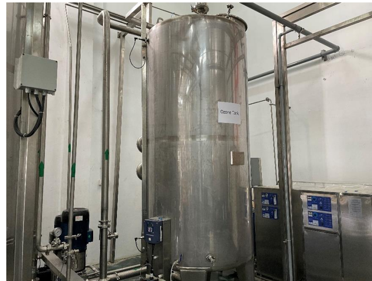
Figure 3-13 Water Purification process Photo in September 6, 2022
