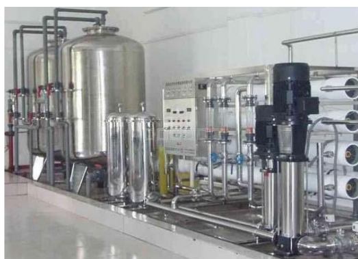
Water Treatment System
