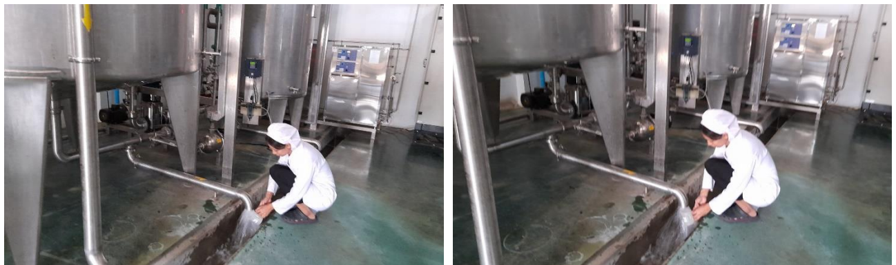
Reject Water/Wastewater Collection Photos
