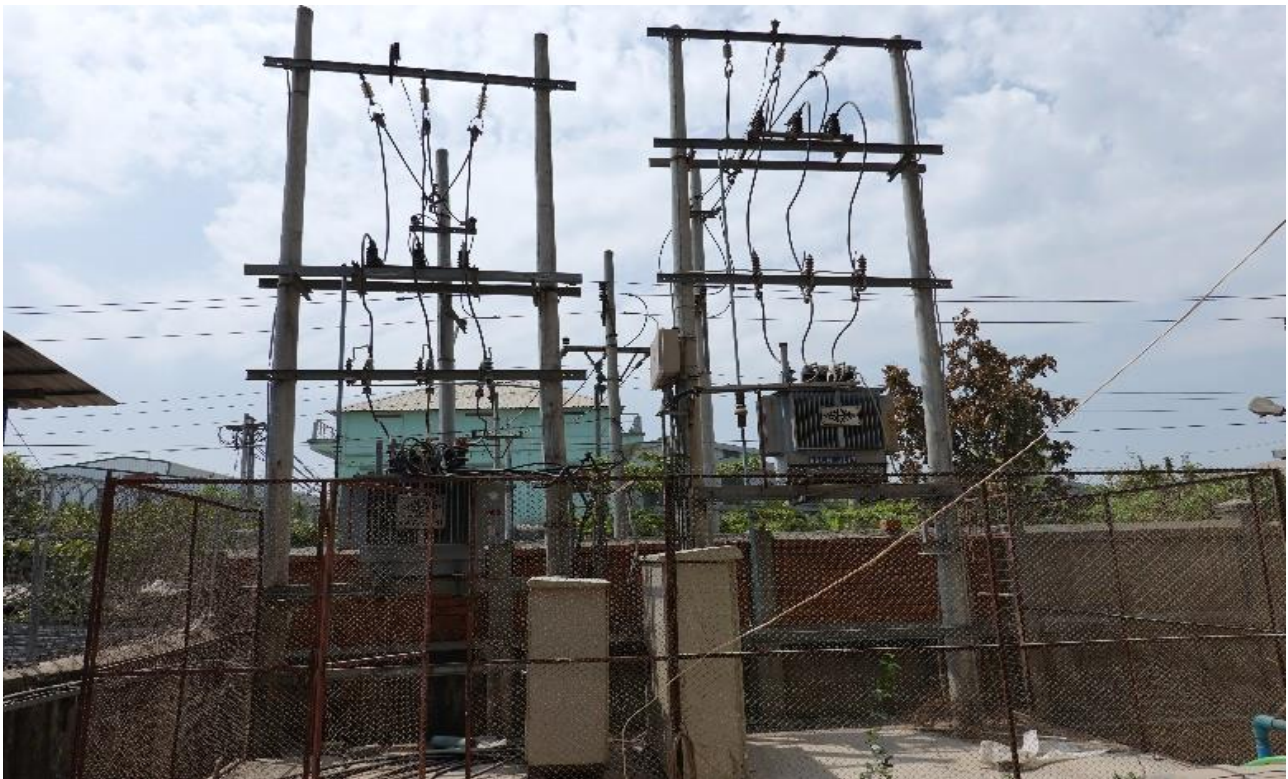
Figure 3-10 Transformers of Proposed Project
