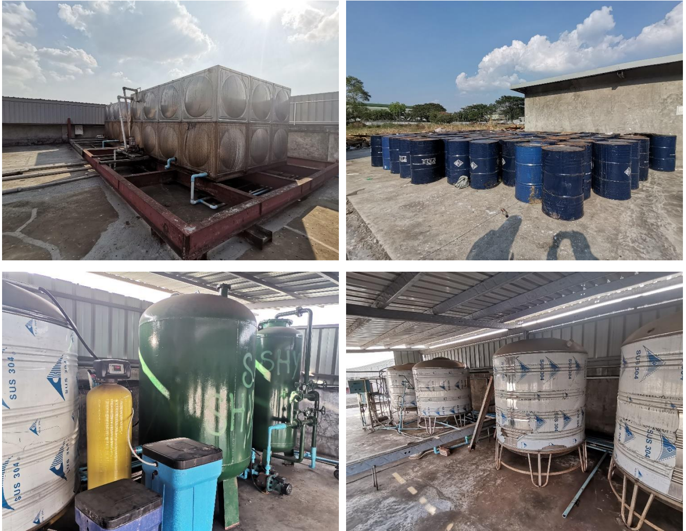
Figure 3-8 Water storage tank supply
