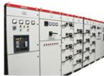
LV incoming cabinet Capacitor compensation cabinet (300kvar)
