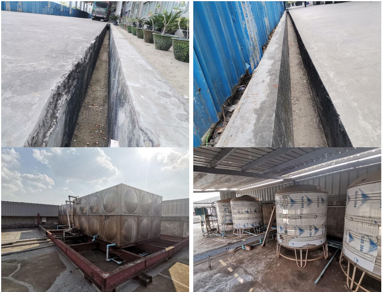
Figure 5-3 Drainage and Septic tank in project area
