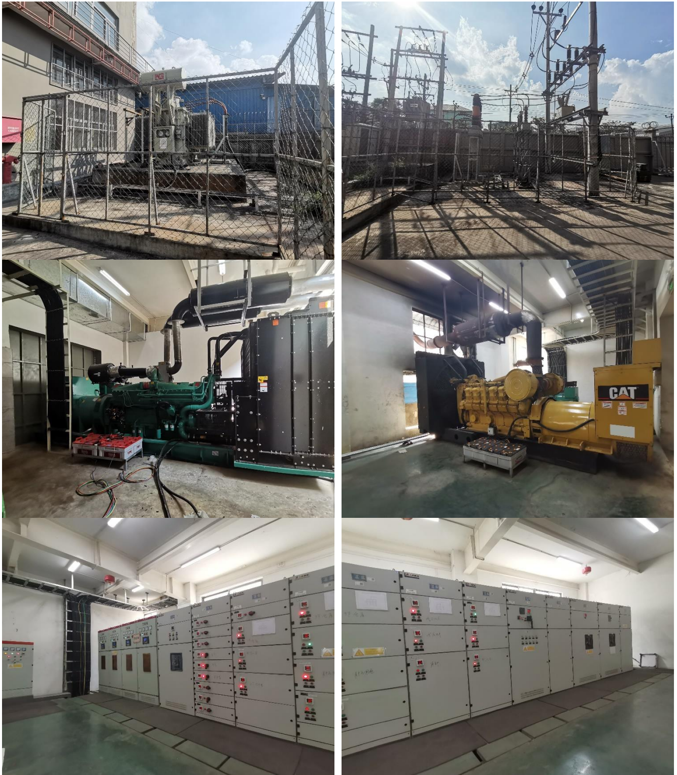
Figure 3-11 Electricity Facilities at Gold Emperor (Myanmar) Factory
