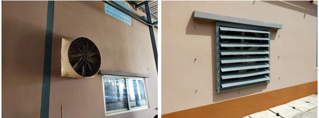
Figure 3-13 Ventilation System at factory
