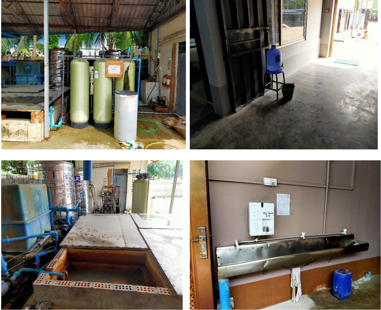
Figure 3-8 Water storage and filtration system
