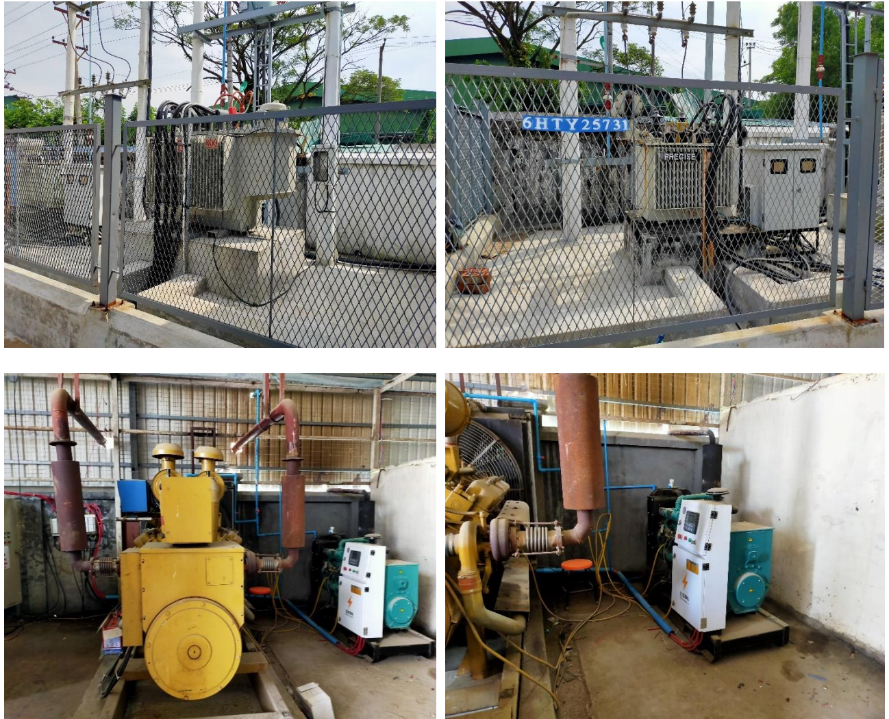
Figure 3-9 Electricity distribution room
