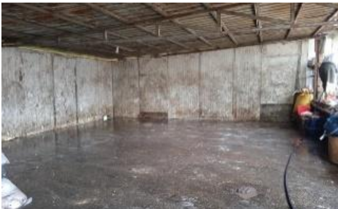
Figure 4.24: Temporary Garbage Tank
