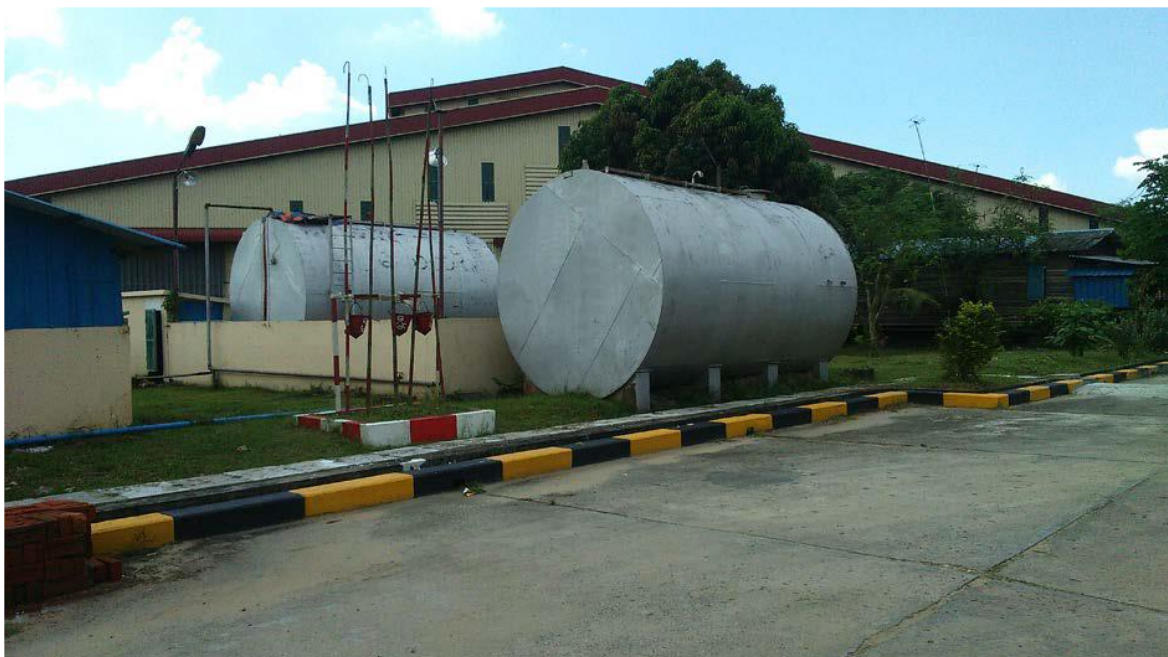
Figure 4.42: Fuel storage tank
