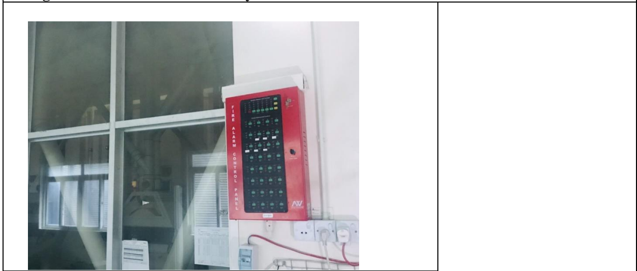
Figure 9.4: Production Fire Alarm System
