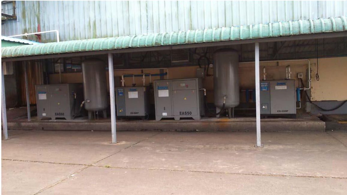
Figure 4.41: Air compressing machines
