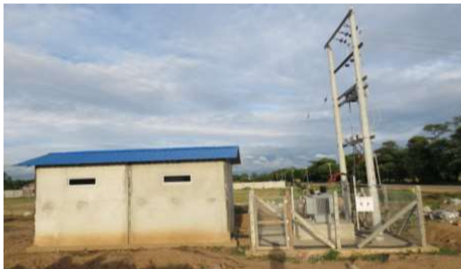
Figure-11: Existing electricity substation
