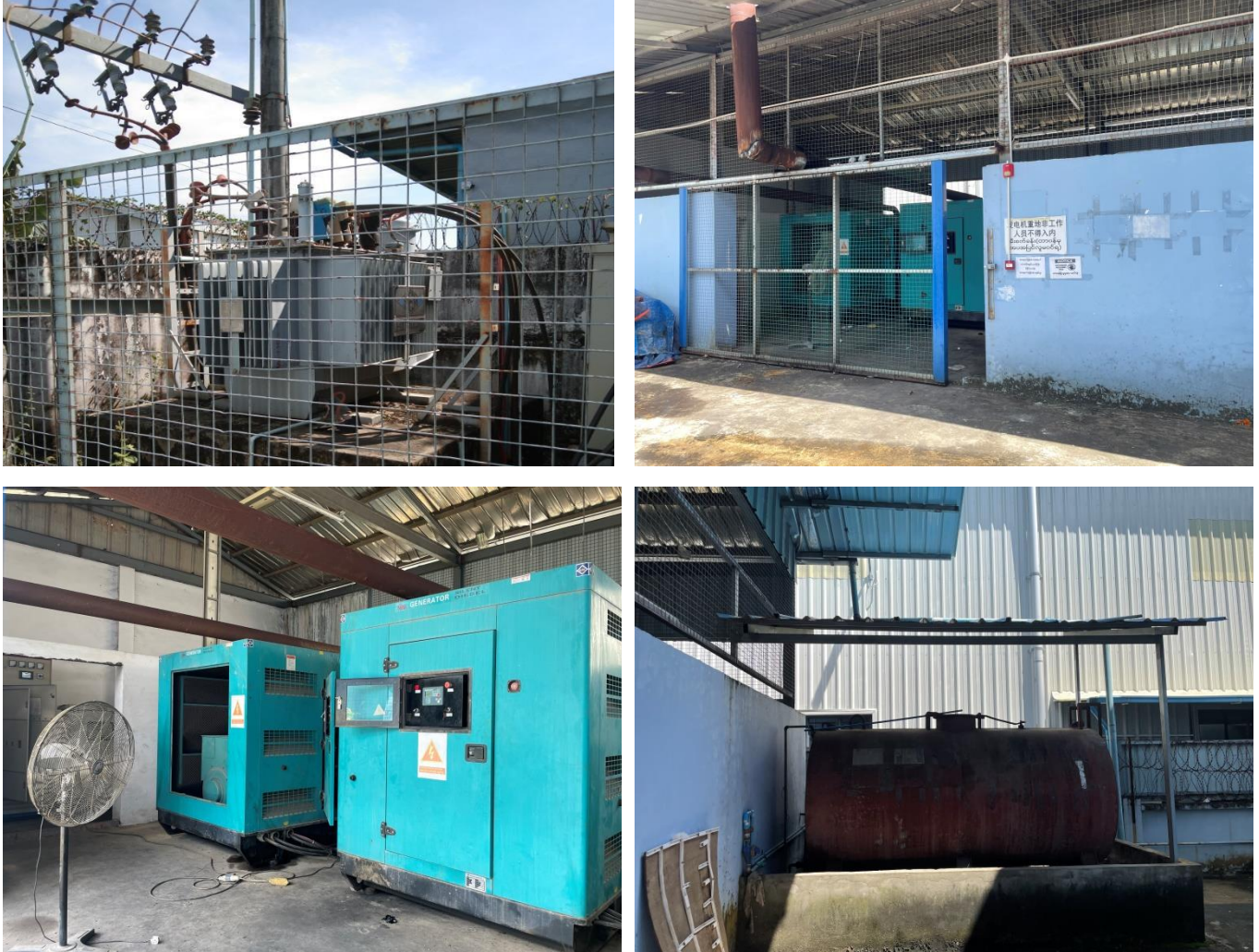
Figure 3-9 Electricity Facilities and Fuel Storage Tank
