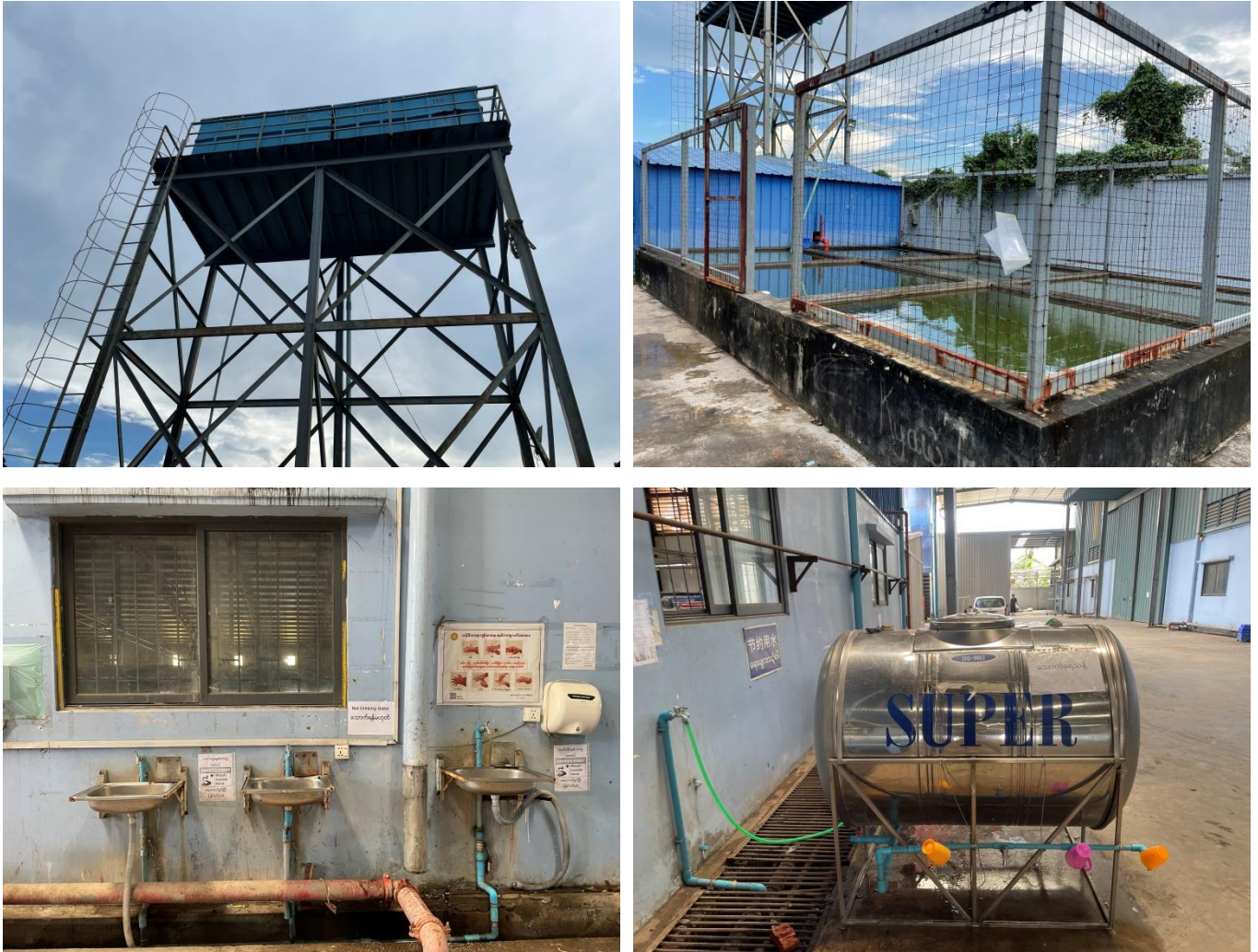
Figure 3-8 Water Storage Tank and Drinking Water Supply
