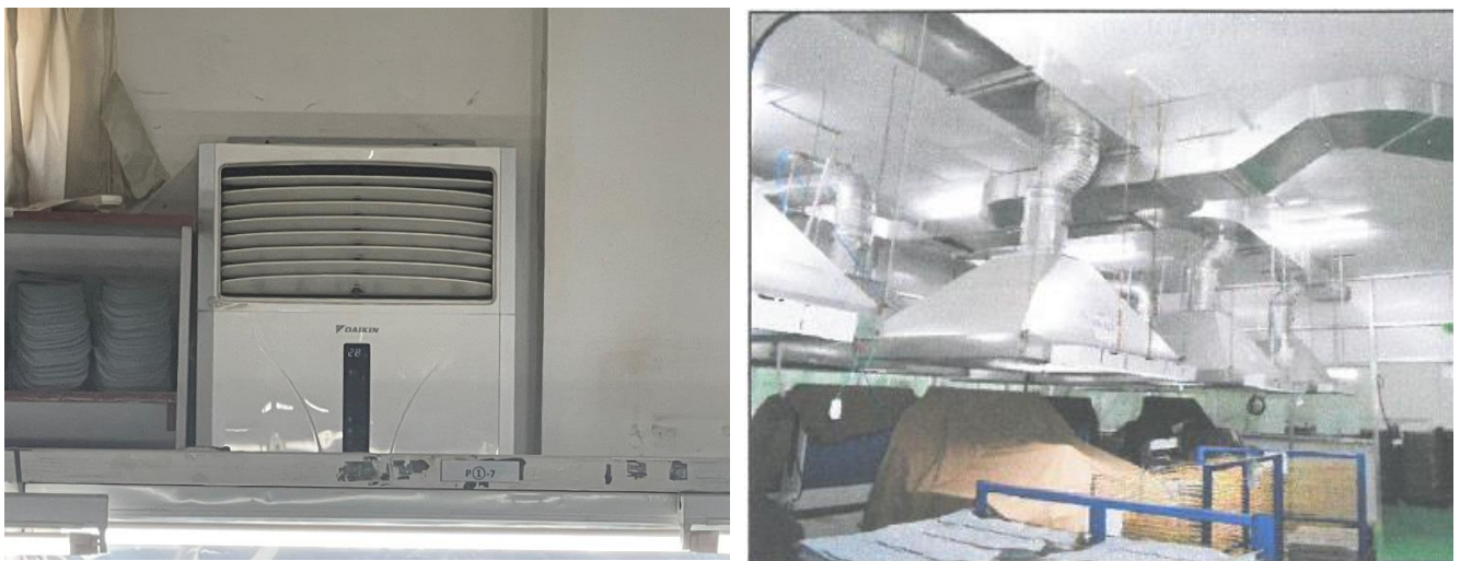
Figure 3-16 Ventilation System Photo
