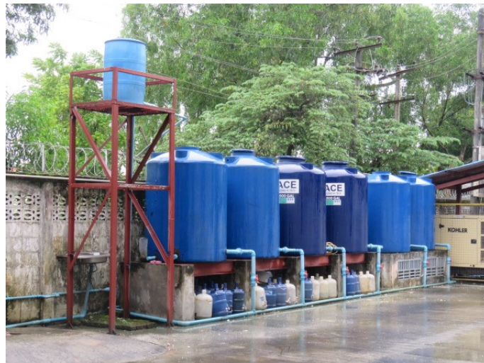
Figur - 34 Elevated tanks
