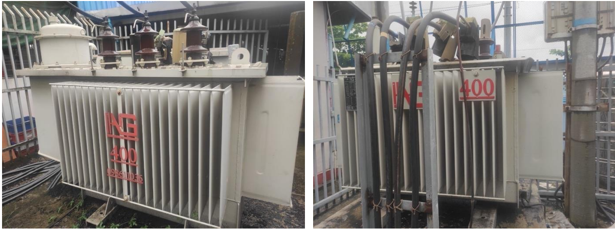
Figure 3.17 National Grid Line to Transformers
