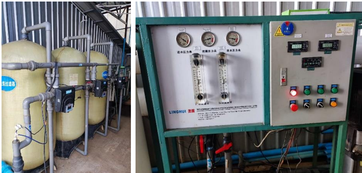
Figure 3.19 Tube Well Water Treatment System for Domestic Use
