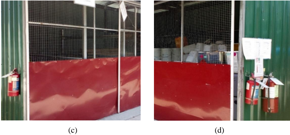
Figure 6.11 (a) – (d) Fire Hose Reel and Fire Extinguishers
