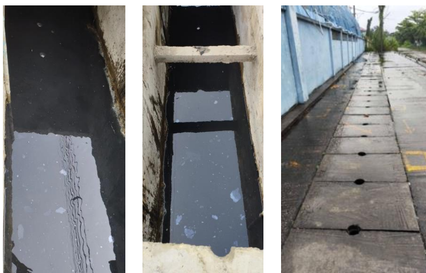
Figure 3.48 Drain System in the Project
