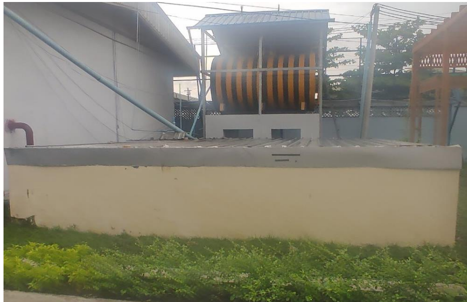
Figure 6.12 Water Tank for Firefighting
