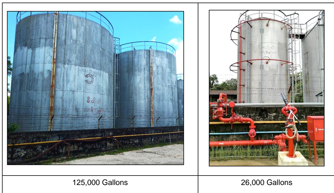
Figure 3-56 Diesel Storage Tank
