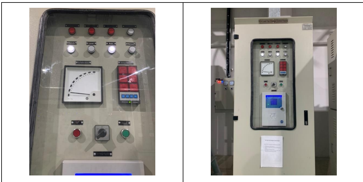
Figure 3-54 Photo of On Load Tap Changer
