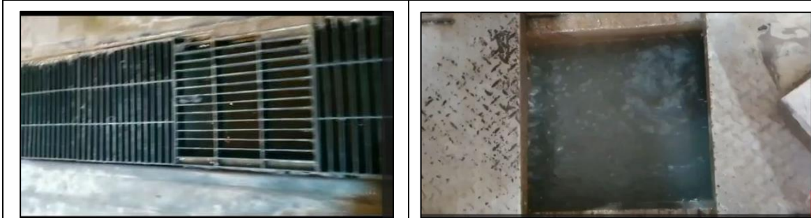
Transfer to Oil Separation Tank
