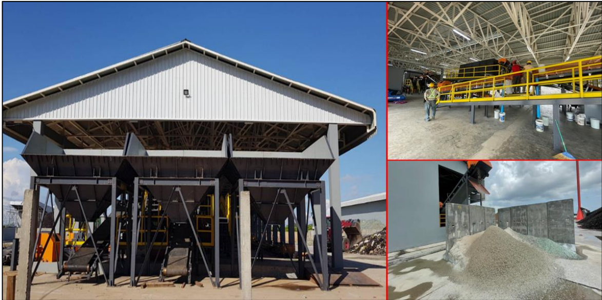
Figure 3-24 Cullet Treatment Plant
