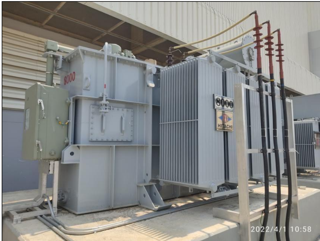
Figure 3-53 Photo of Transformer
