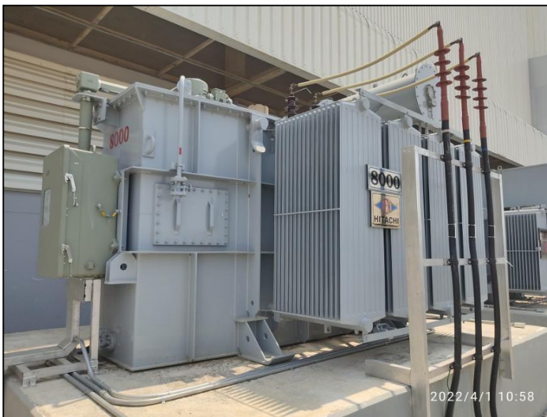
Figure 9 Photo of Transformer
