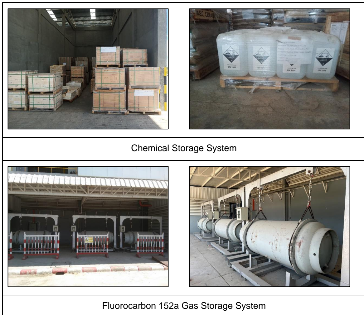
Figure 7-4 Chemical Storage Condition
