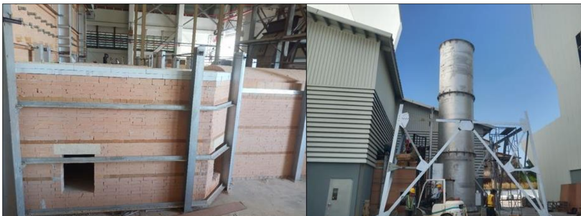
Figure 3-29 Furnace and Chimney
