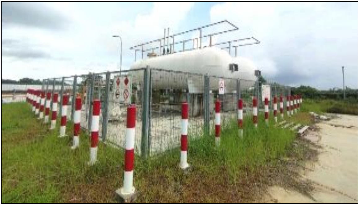
Figure 3-57 LPG Storage Tank
