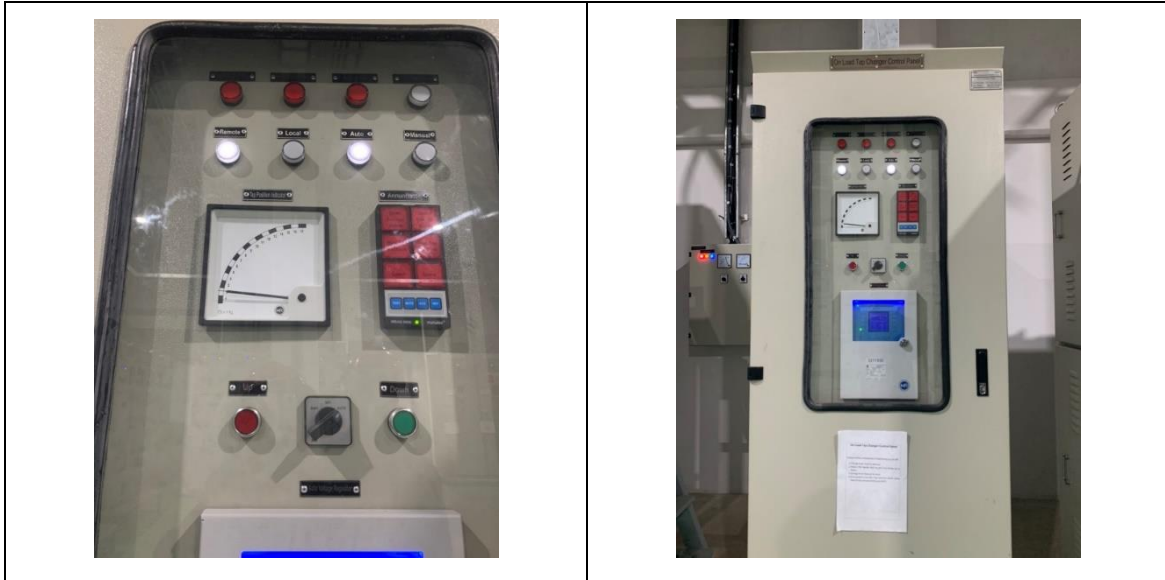
Figure 10 Photo of On Load Tap Changer
