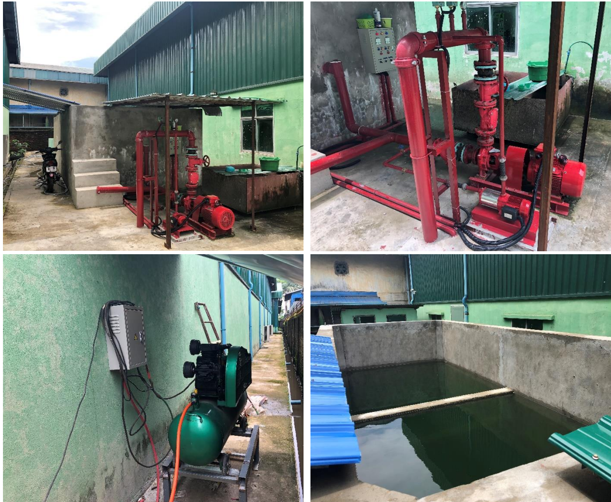
Figure 3-11 Water storage and filtration system
