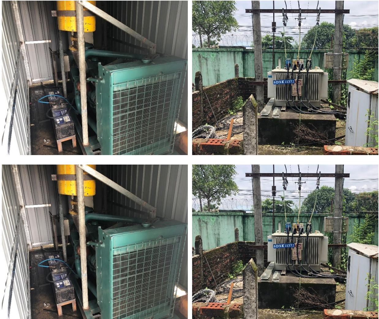
Figure 3-13 Electricity distribution room
