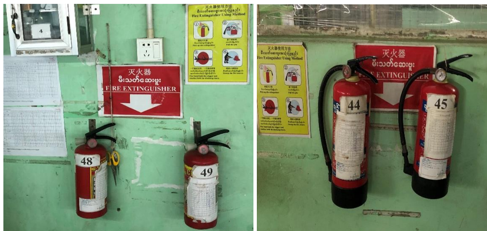
Figure 7.2 Photos of Facilities for Fire Prevention
