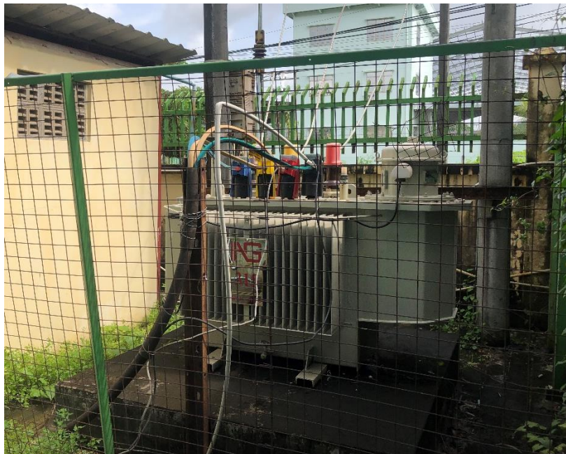
Figure 3-12 Photo of Transformer
