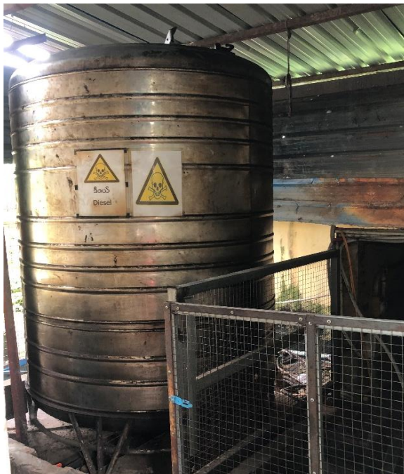
Figure 3-14 Photos of Diesel Fuel Storage for Generators
