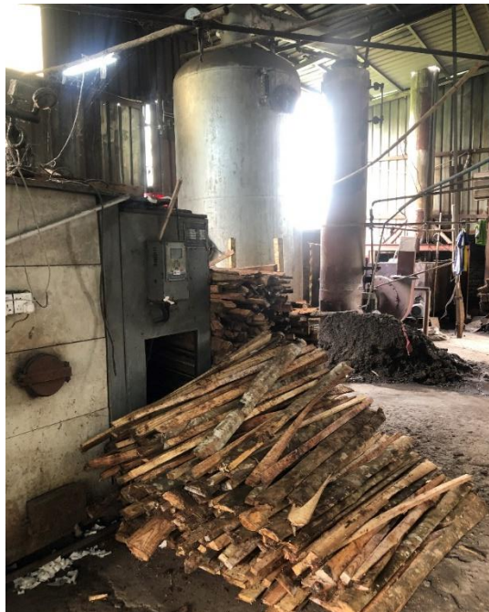
Figure 3-16 Photo of Boiler
