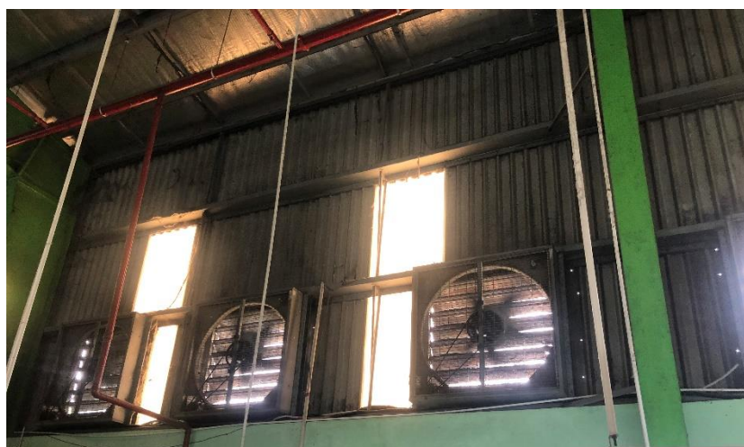
Figure 3-20 Photo of Ventilation
