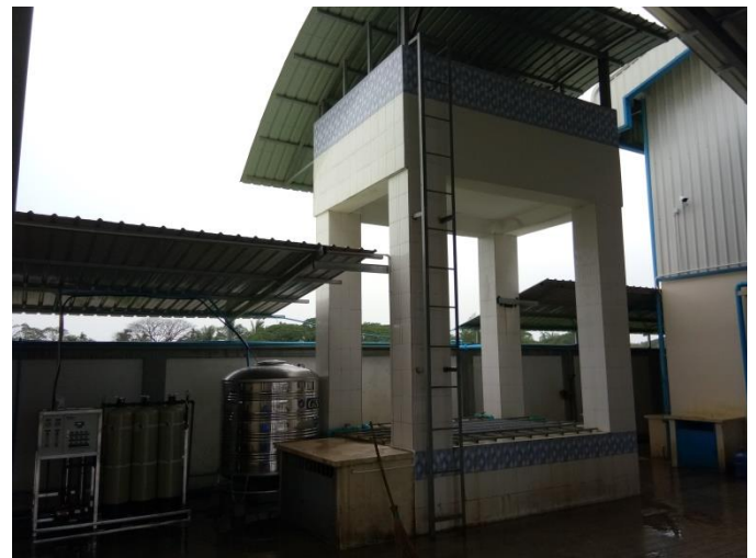
Overhead and ground water tank
