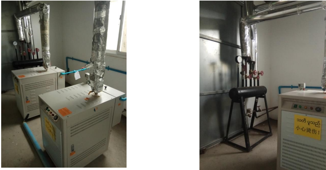
Figure 3-9 Electronic Steam Boiler at Xiang Rui Factory
