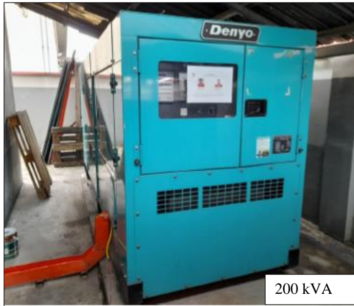
Figure 3.17 Generators at Factory
