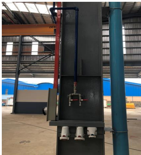
Figure 5.6 Photo of Compressed Air Pipe Line
