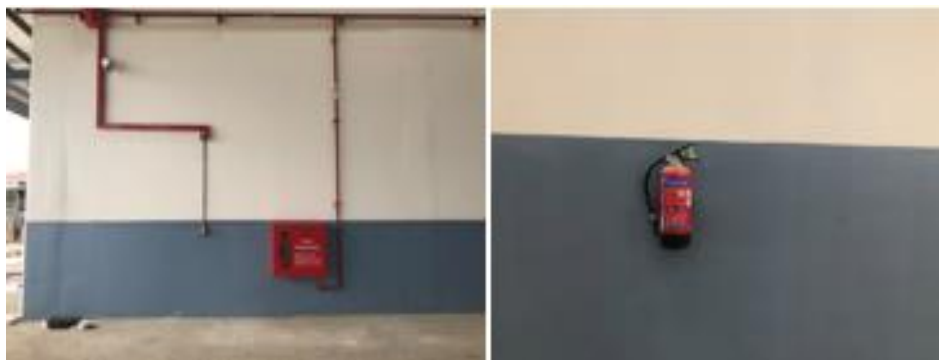
Figure 5.7 Fire Fighting System
