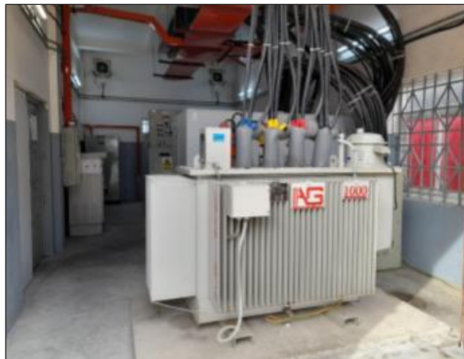
Figure 3.16 Transformer at Factory
