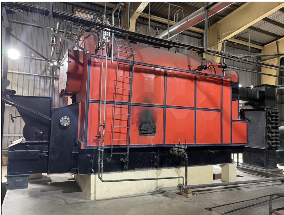
Figure 3-28 Current Boiler Installation at the Factory
