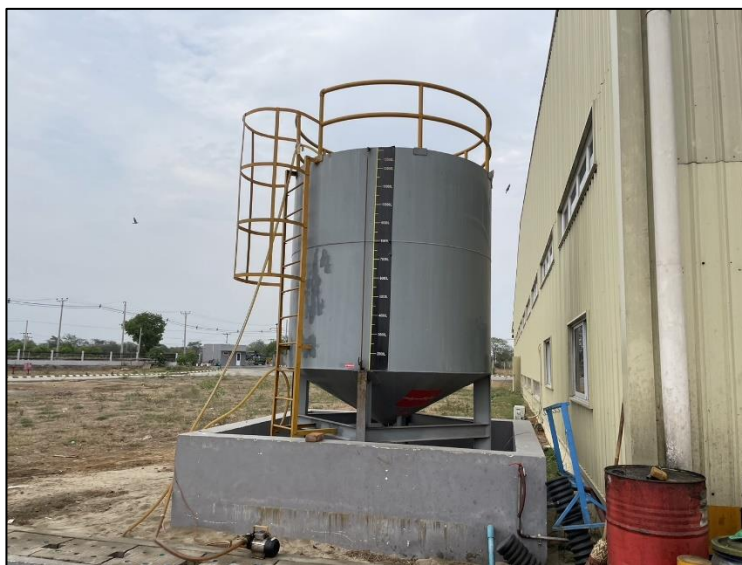
Figure 3-26 Fuel Storage Tank
