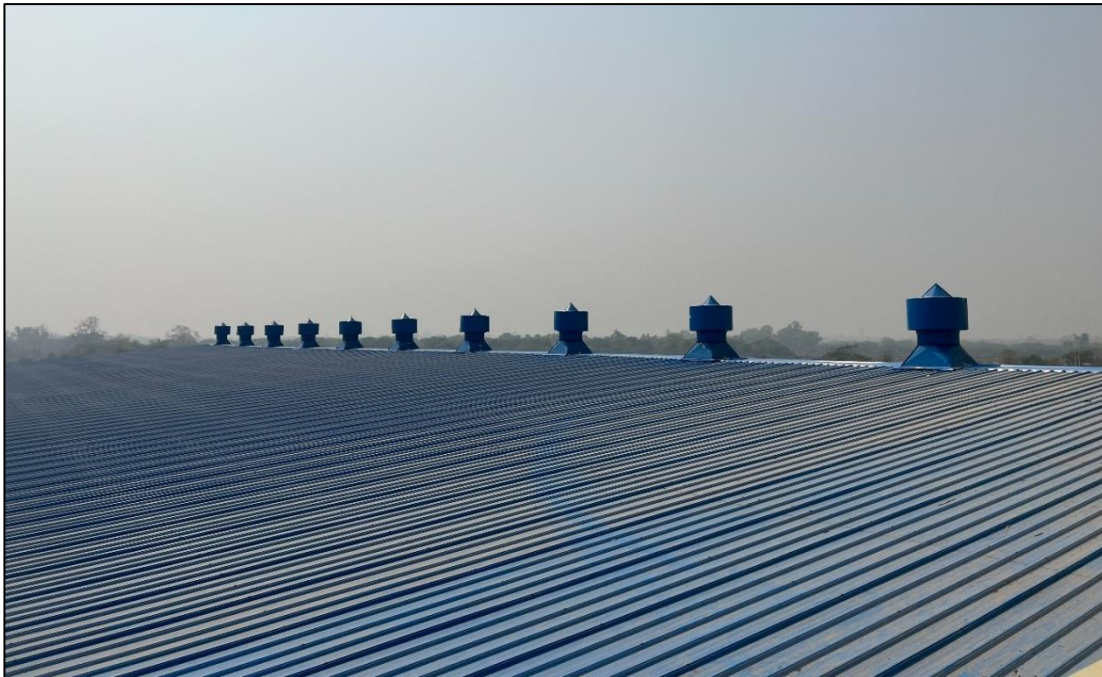
Figure 3-21 Roof Ventilation Fan
