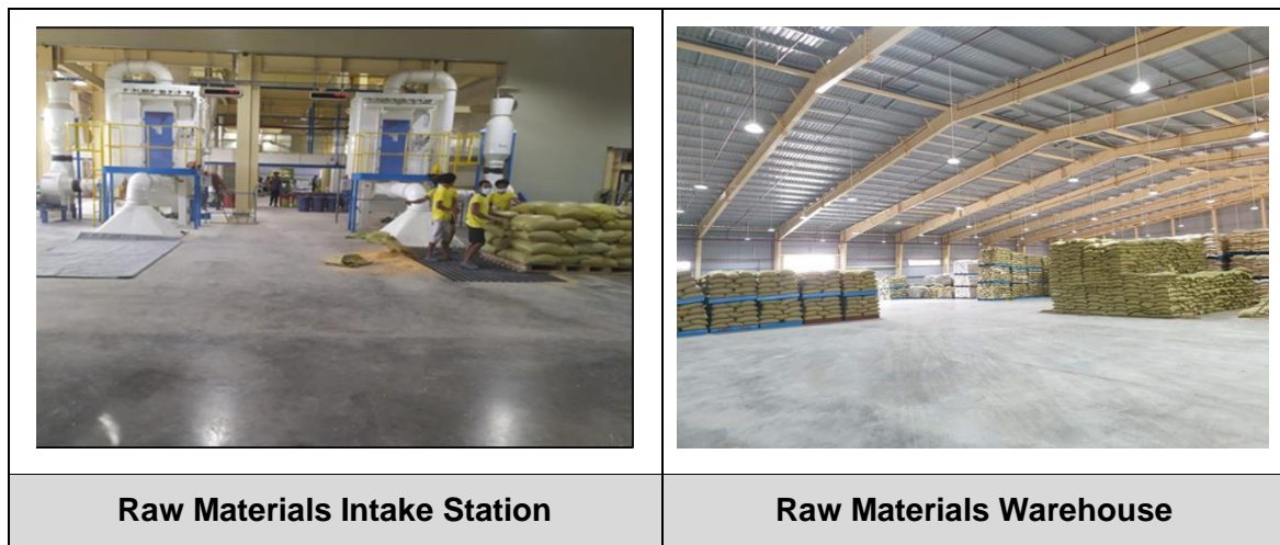
Figure 3-13 Raw Materials Intake Station and Raw Materials Warehouse
