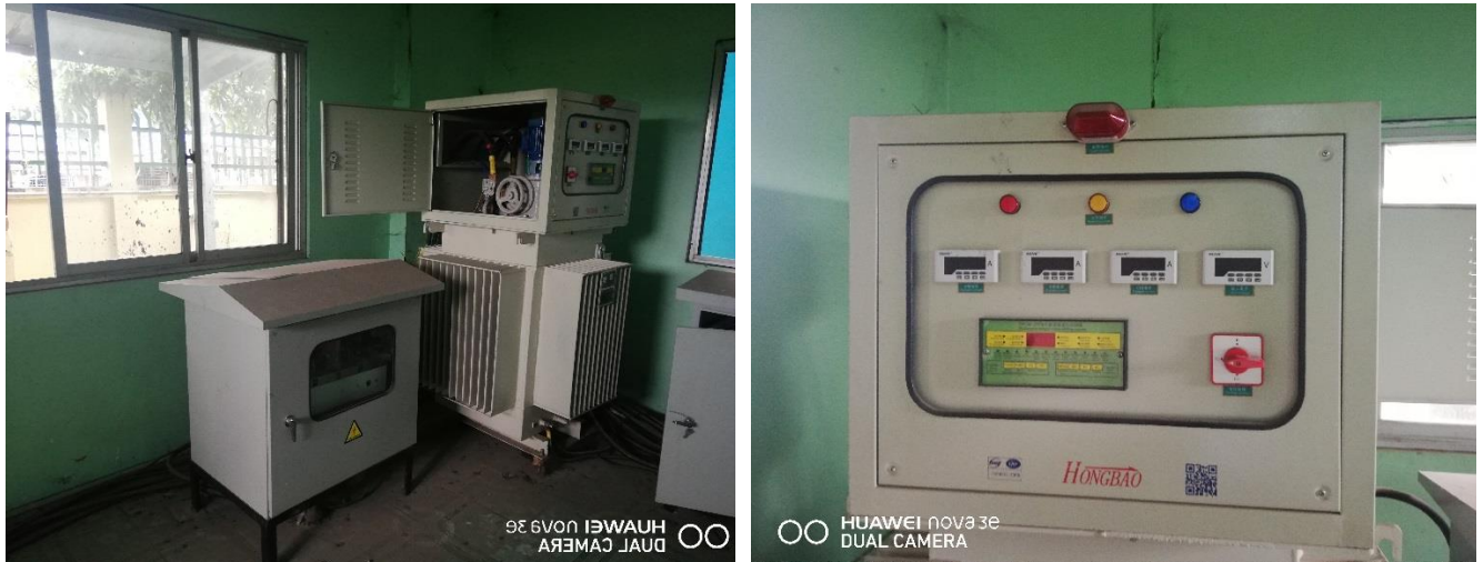
Figure 3-2 Electricity facility at Sunme (Myanmar) Industrial Limited
