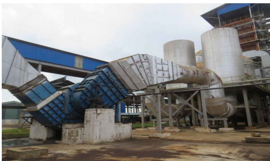
Figure – 71: Dust collector and ID fan
