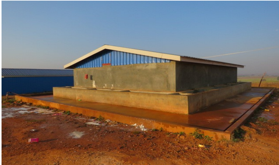
Figure-45: One of five the concrete water tanks for family line
