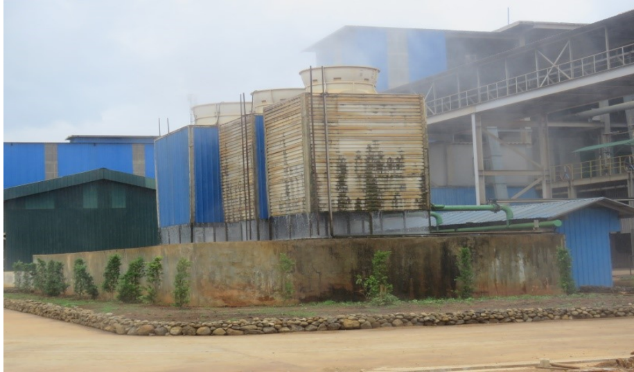
Figure – 24: Cooling Tower
