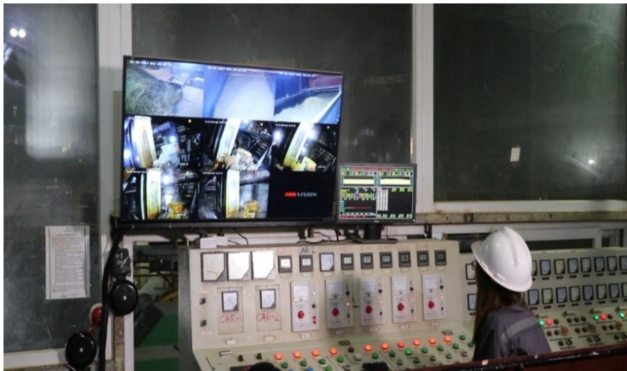
Figure-56: Control room
