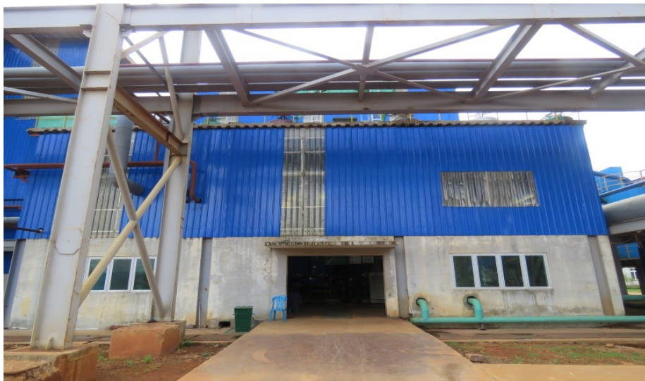
Figure – 23: Boiler House
