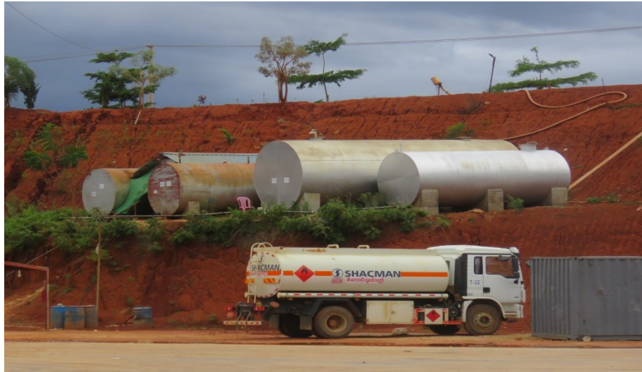
Figure-46: Fuel depot
