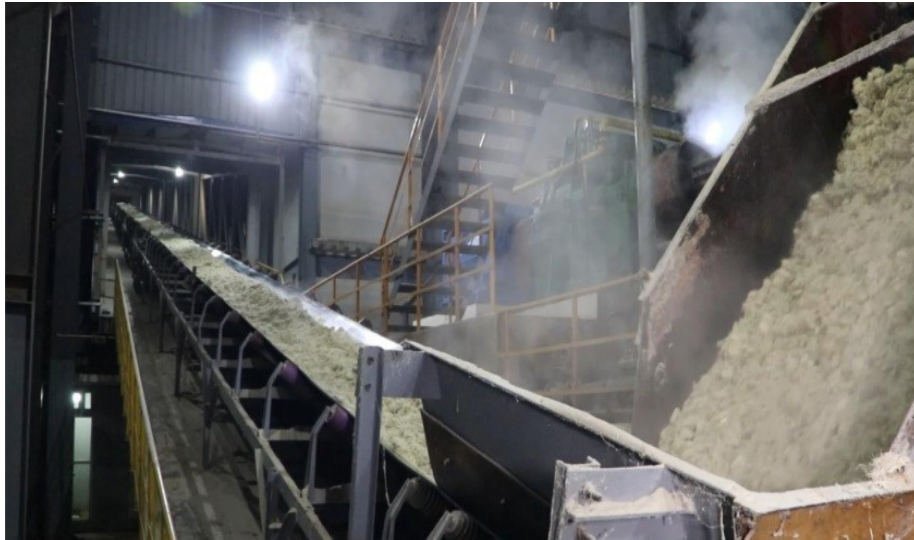
Figure-55: Conveying bagasse to boiler unit
