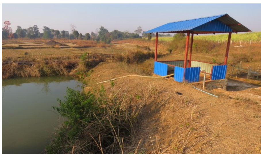
Figure-42: Underground spring and pump house (the water is distributed to Hsen Taw village)
