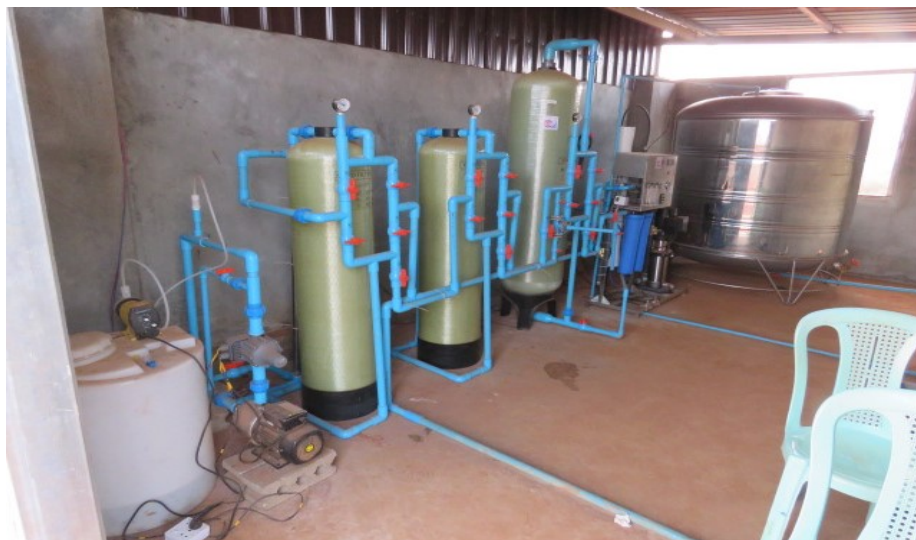
Figure-44: Water purification system
