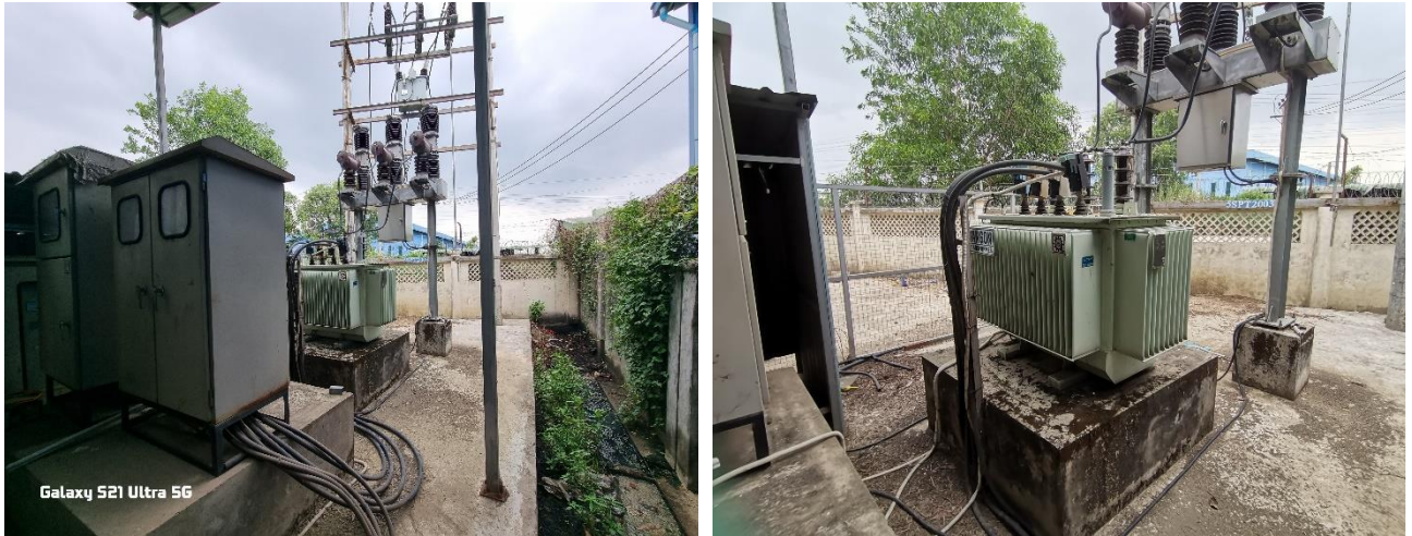
Figure 3-7: Transformer and Generator in the Factory
