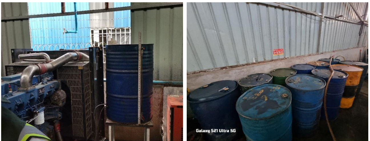
Figure 3-8: Storage Tank for Fuel
