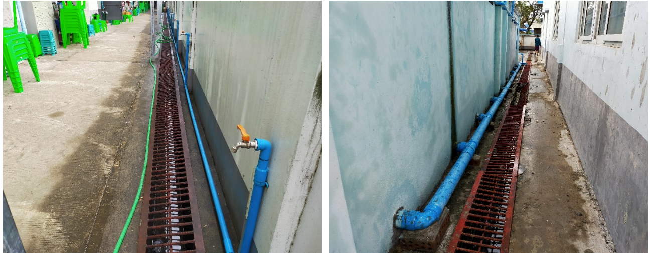
Figure 3-9 Rainwater Drainage in the factory compound
