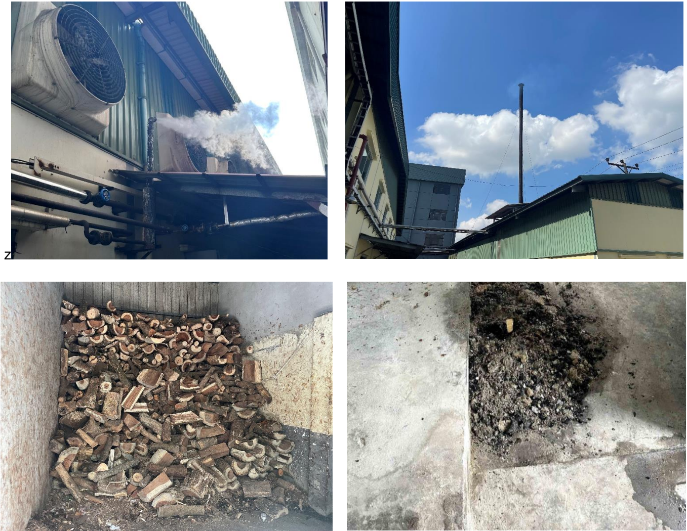
Figure 2-3 Steam Boiler at Zong Hong (Myanmar) Garment Factory
