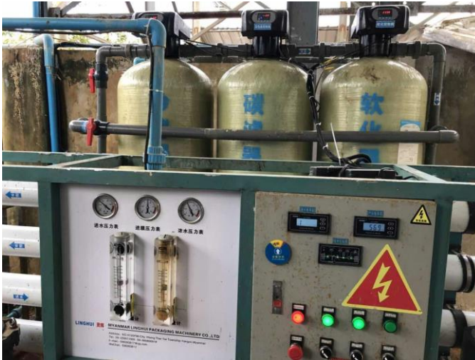
Water Filtration System
