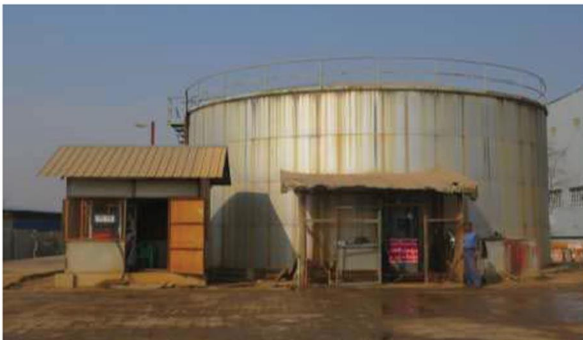
Figure 3-24 Photo of Oil Storage Tank
