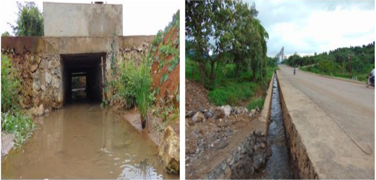
Figure 3-28 Drainage System of the Cement Factory
