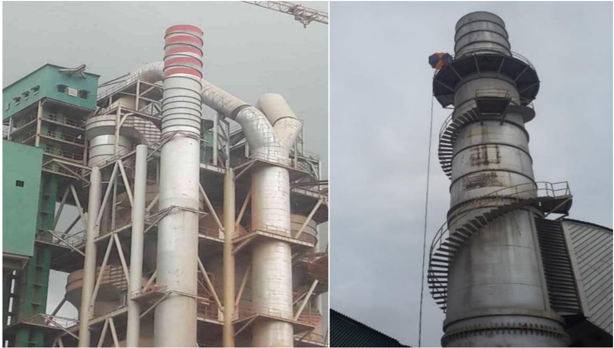
Figure 3-21 Example of Preheater Stack and Cooler Stack
