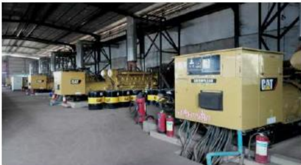
Figure 3-23 Photo of Stand by Diesel Generator
