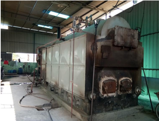
4 tons of Steam Boiler
