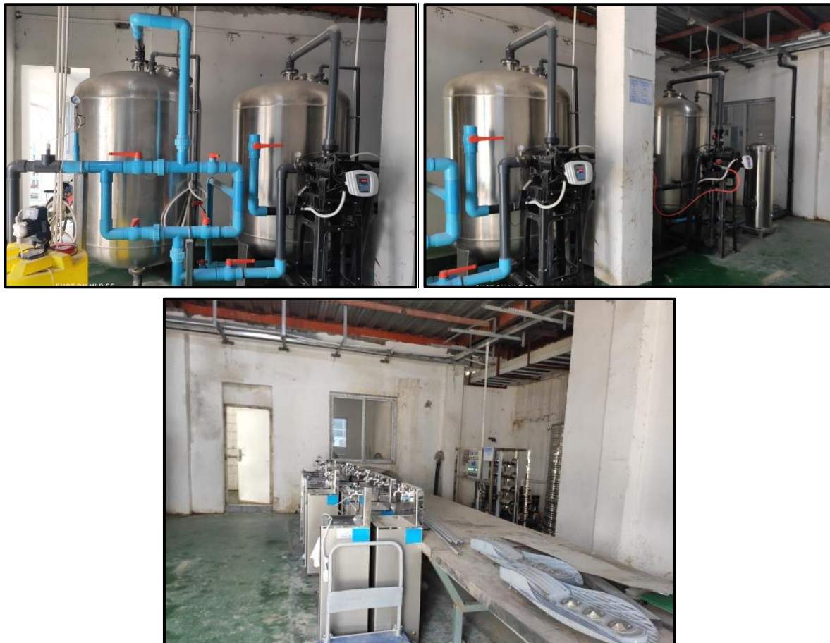
Figure 3-11 Photos of 2T/H RO Pure Water Treatment Tanks
