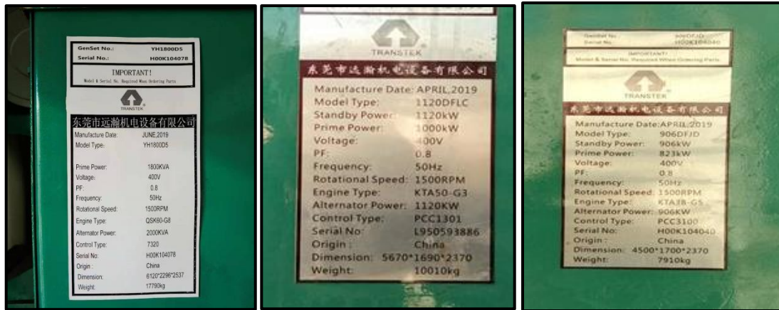
Figure 3-8 Generators at Factory
