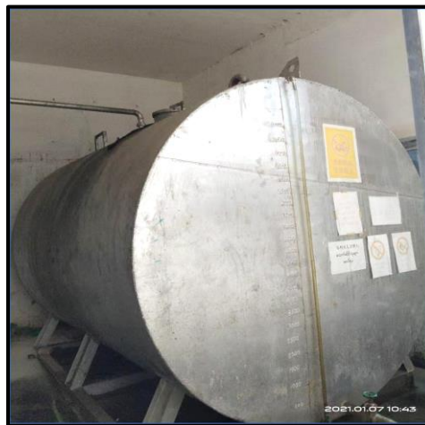
Figure 3-9 Diesel Storage tank
