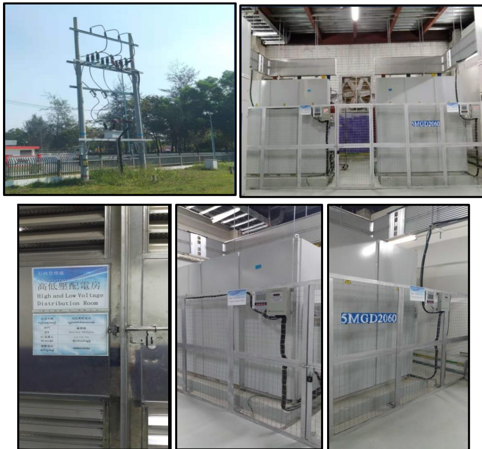
Figure 3-7 Transformers at Factory
