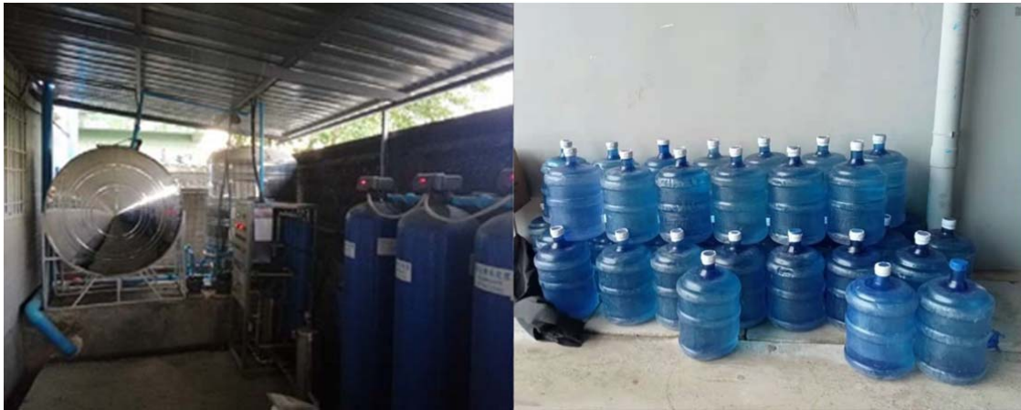
Figure 1-8 Water storage and filtration system
