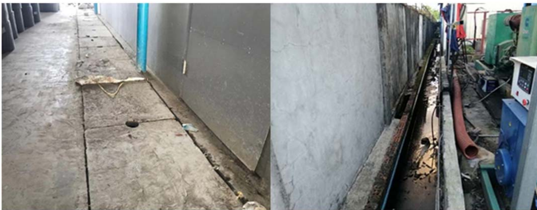
Figure 1-9 Rainwater drainage in factory compound
