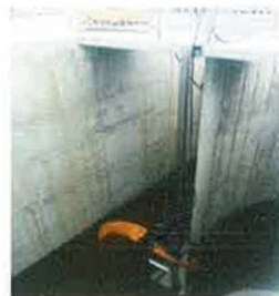
The Whole Equipment (Anaerobic Treatment)
