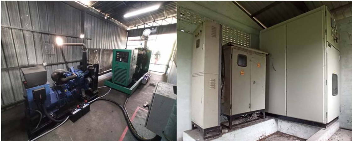
Figure 1-10 Electricity distribution room
