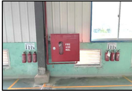
Figure 9-3 Some Fire Extinguishers in the Factory
