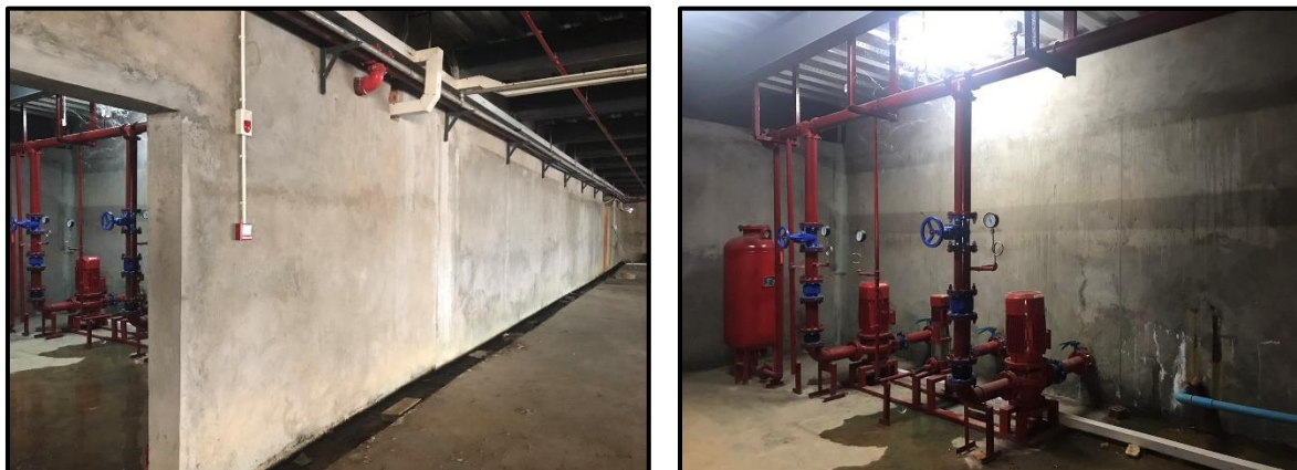
Figure 9-5 Water Storage Tank and Machine for Fire Fighting
