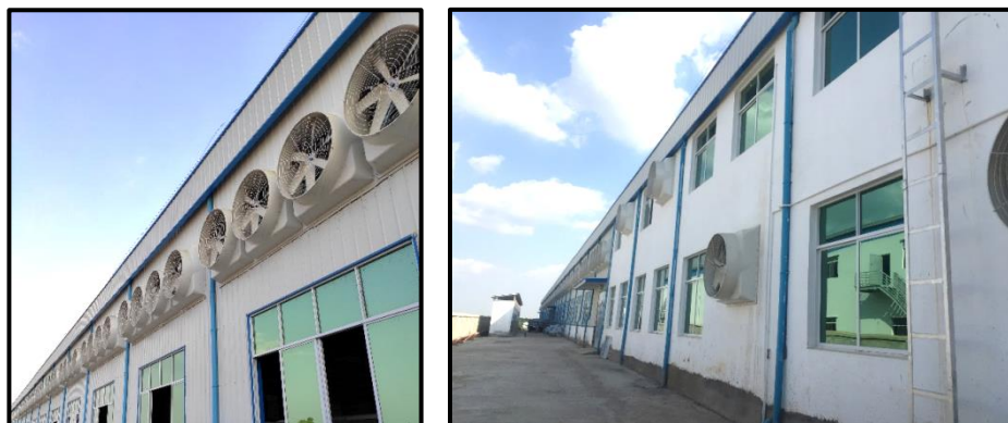
Figure 5-4 Installed Air Extraction Fans
