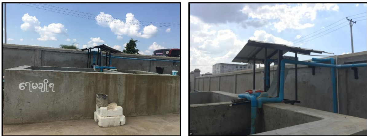
Figure 2-28 Water Storage Tanks for Domestic Use
