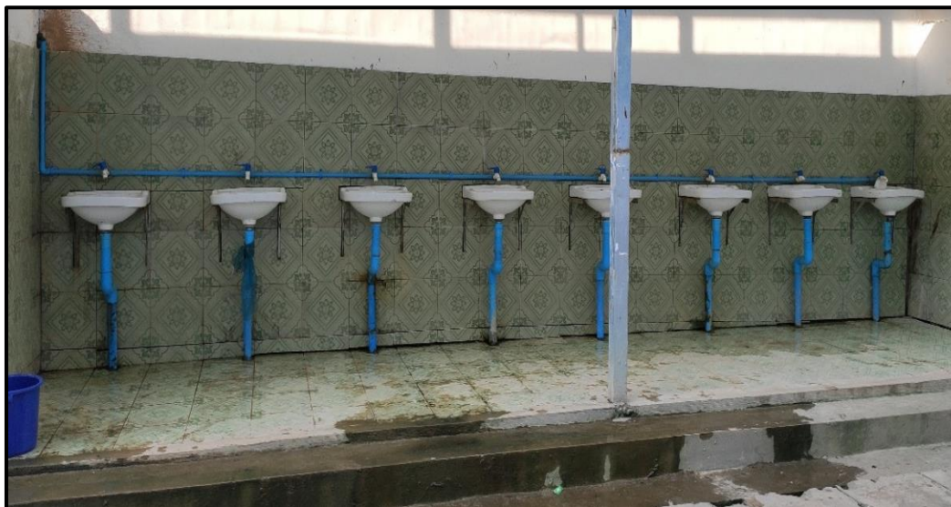
Figure 2-29 Water Taps for Domestic Use
