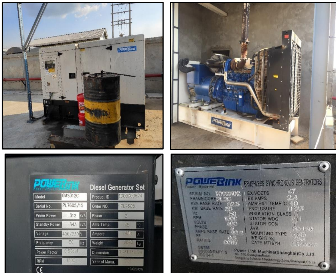
Figure 2-24 Generators Used in Factory
