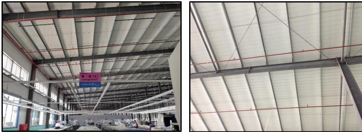
Figure 9-4 Fire Sprinklers in Factory
