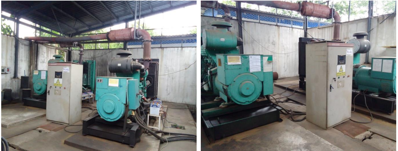
Figure 3-11 Electricity distribution Room and Generator Room
