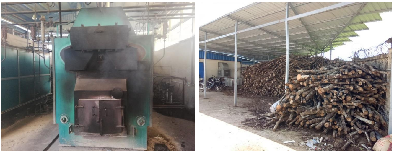
Figure 3-12 Steam boiler and firewood fuel
