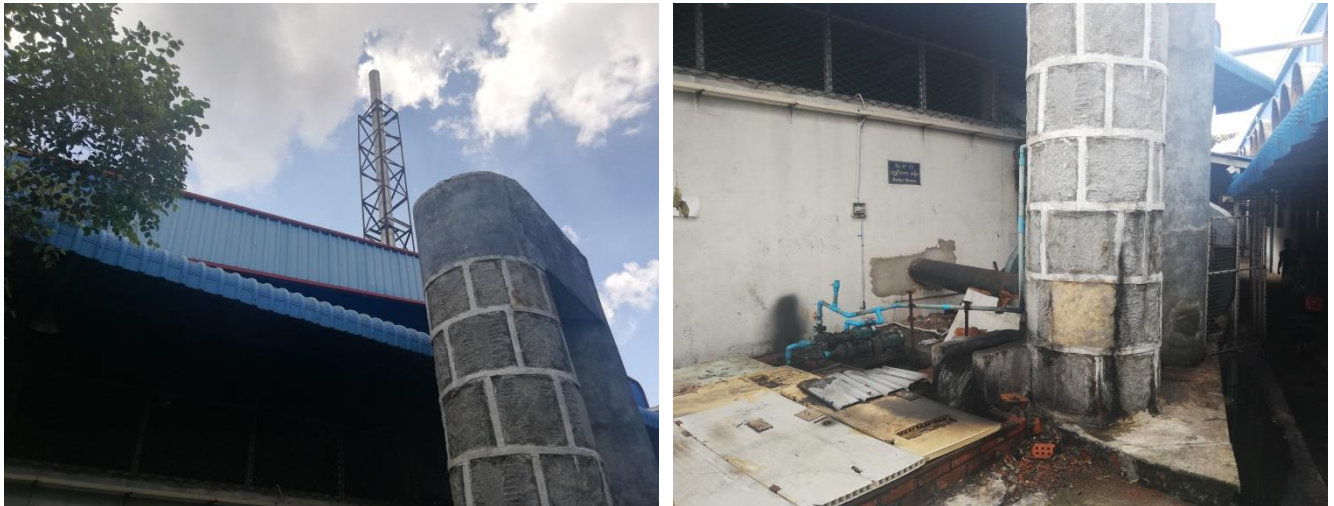
Figure 3-13 Chimney photo of boiler
