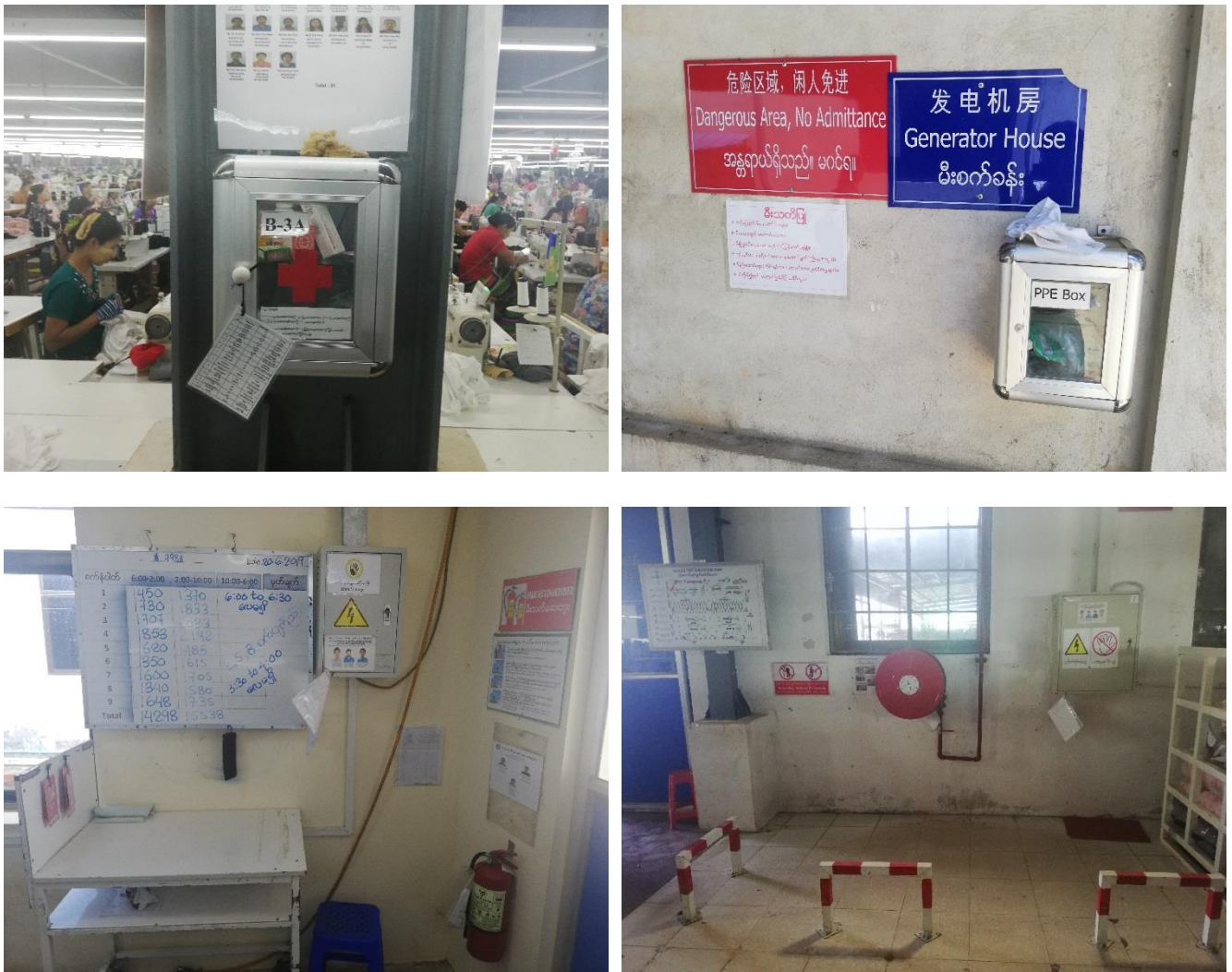
Figure 3-3 Fire Safety facilities
