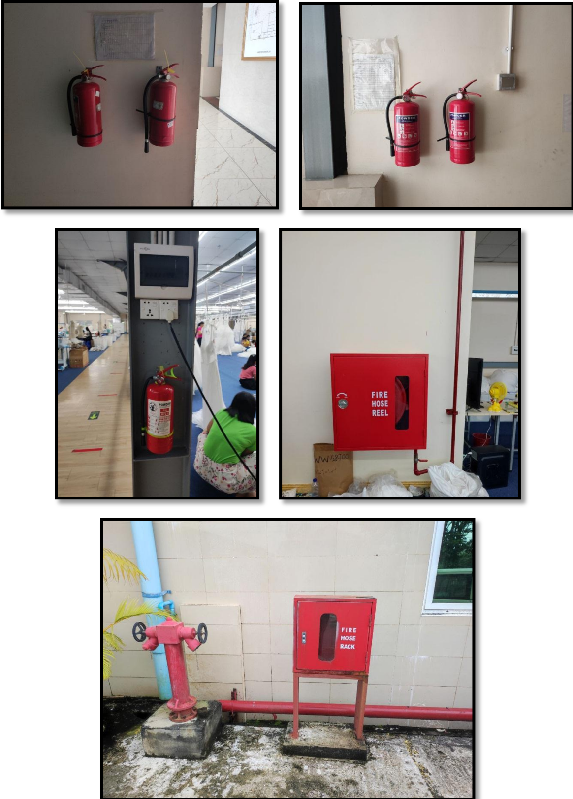
Figure 7-2 Photos of Extinguisher and Fire Tank
