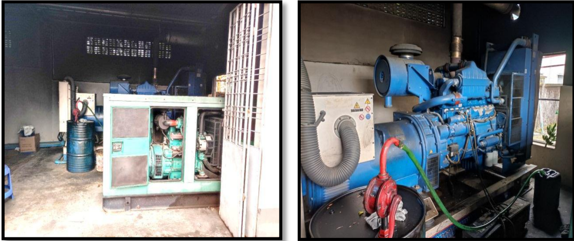
Figure 3-12 Photos of Generator and Transformer
