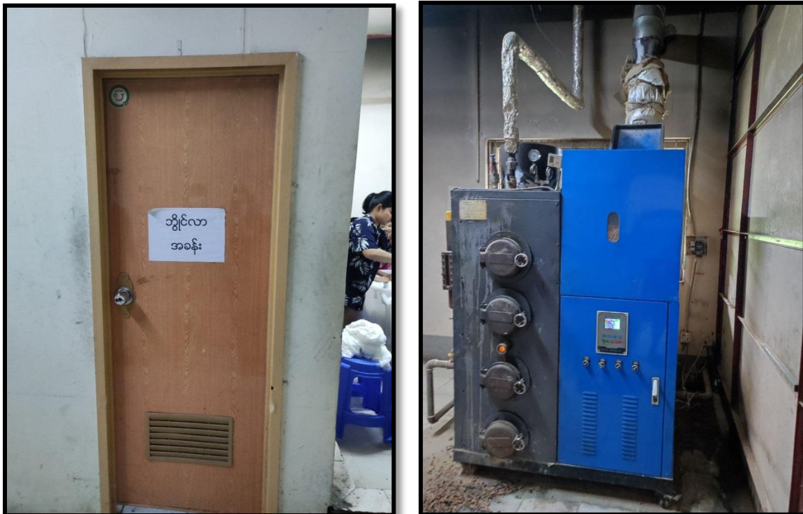
Figure 3-14 Photos of Boiler for Ironing Section and its fuel
