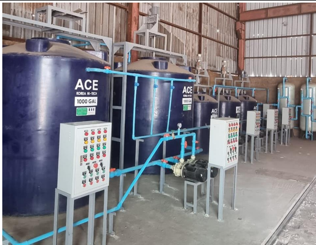
Figure 3.17 Wastewater Treatment Plant
