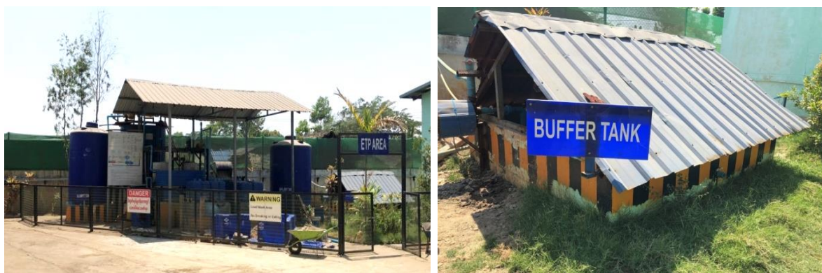
Figure 3.14 Effluent Treatment Plant in MYSARCO Factory
