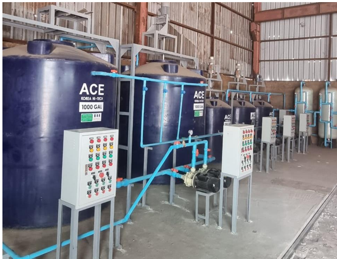
Figure 7.9 Wastewater Treatment Plant
