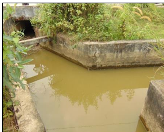
Industrial Drainage Channel
