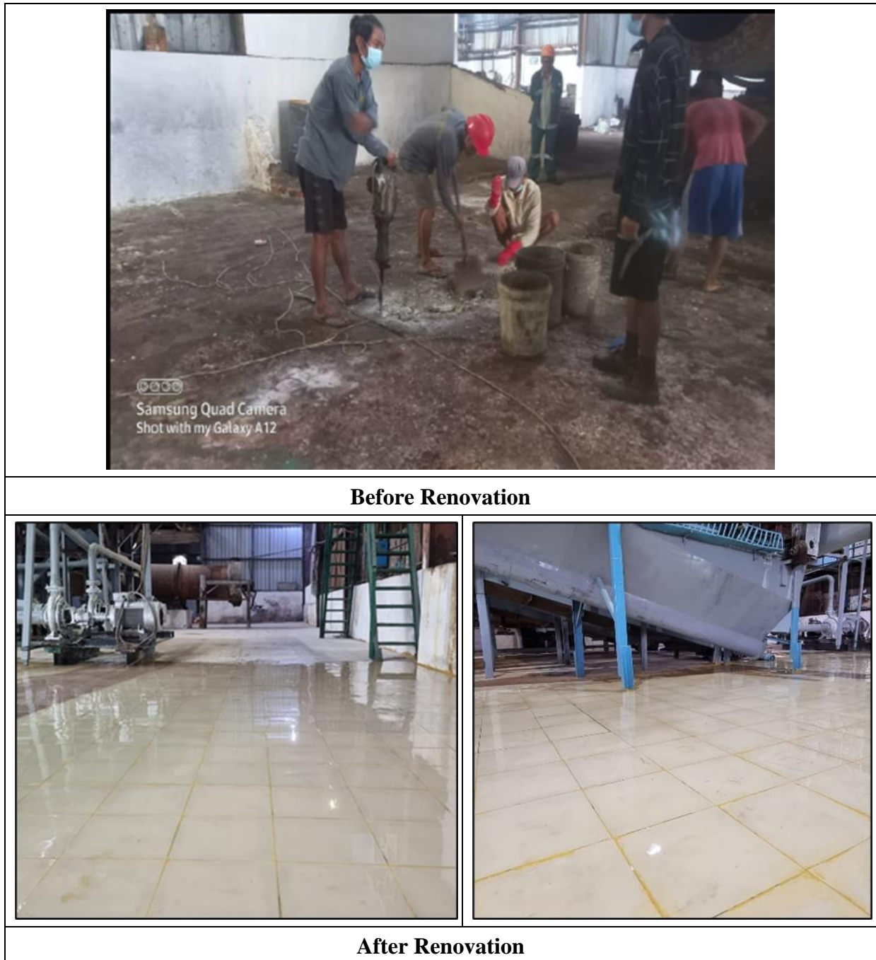
Figure 3.32 The Floor of Batteries Breaking Unit Area (Current condition as of October 2023)
