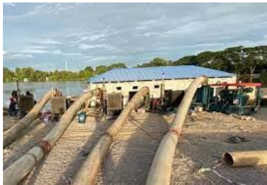
Shwege Stormwater pumping station 6
