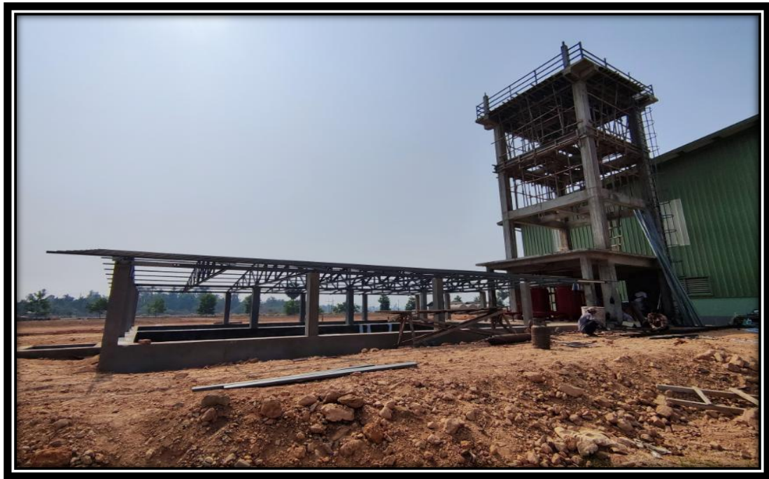
Figure 4.20 Over Head Tank
