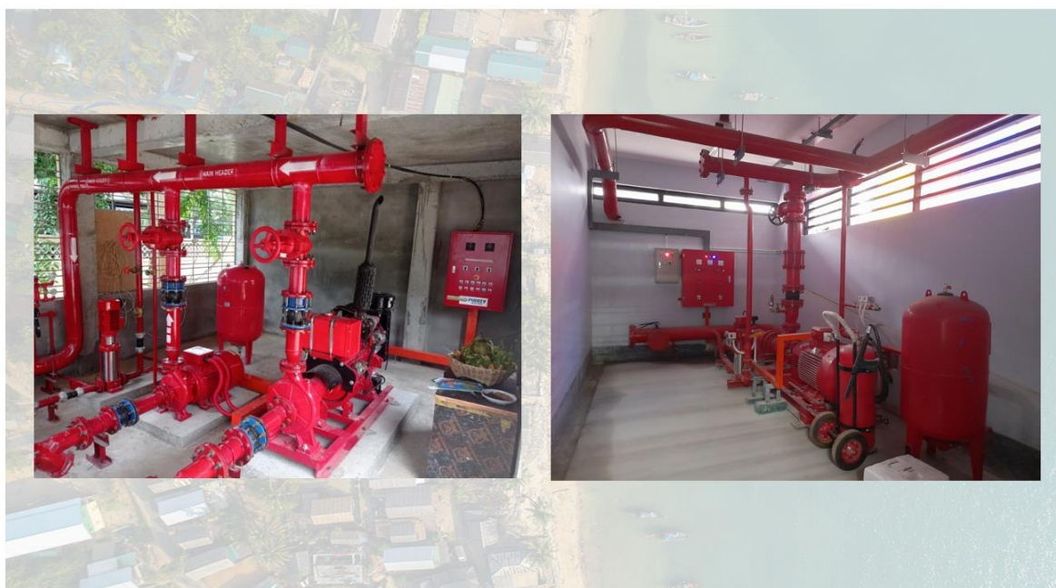
Figure 8.7 Pump house for fire water
