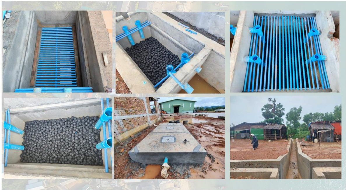
Figure 8.4 Waste water treatment plan septic tanks
