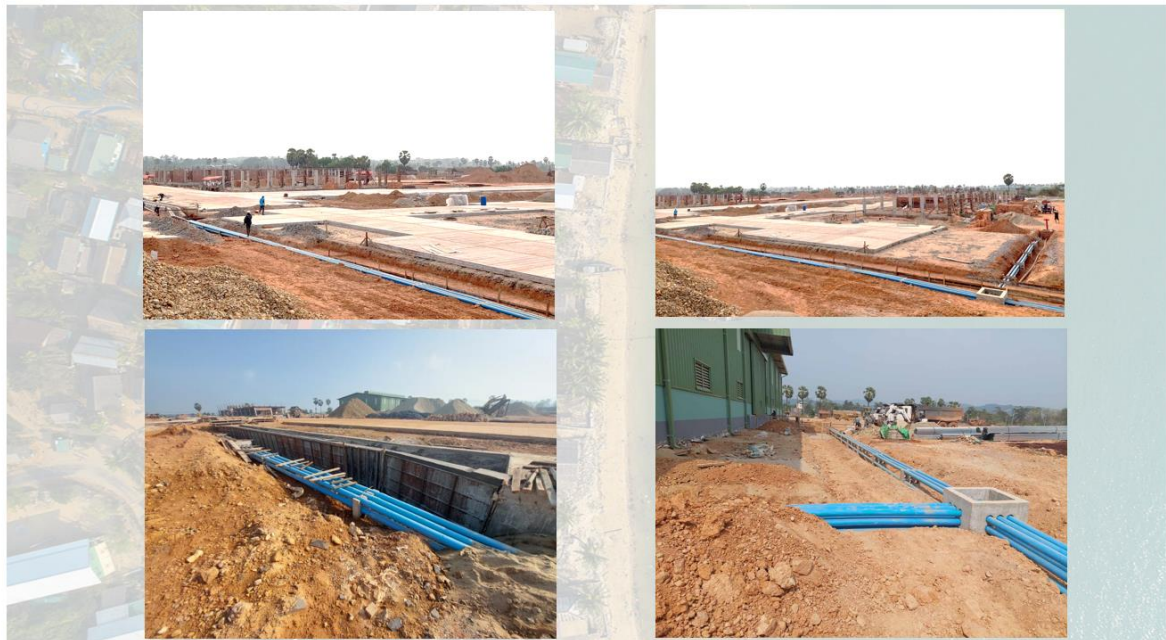
Figure 4.36 Underground water pipe line images
