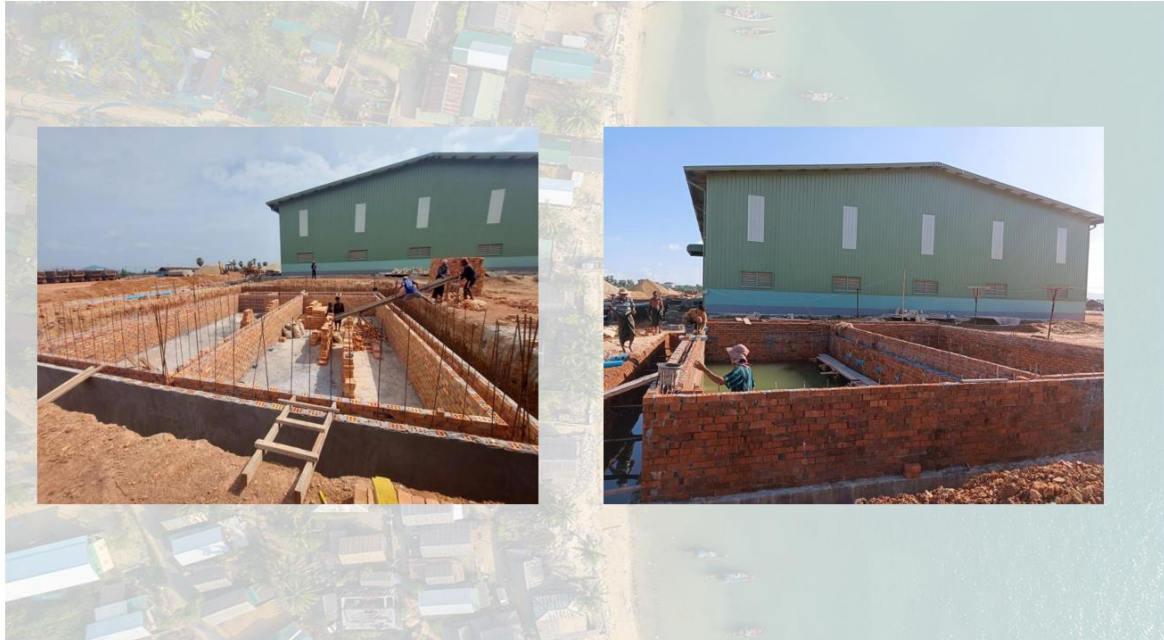
Figure 4.37 Current images of 7000 capacity groundwater tank
