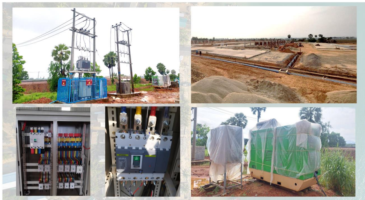
Figure 4.39 Electrical System in project site
