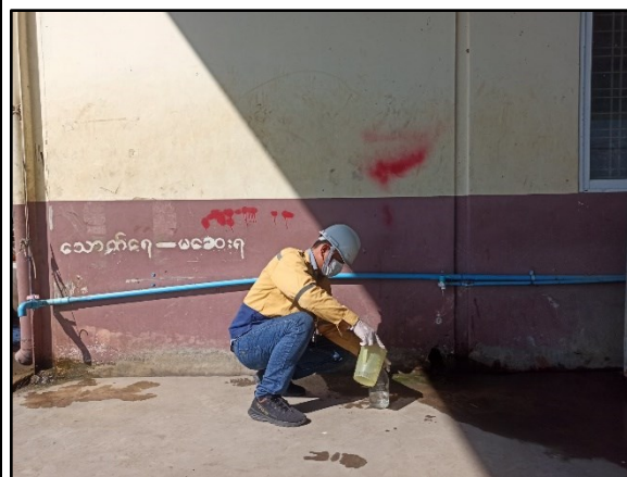
Drinking Water Treatment Plant (P 1) Dry Season
