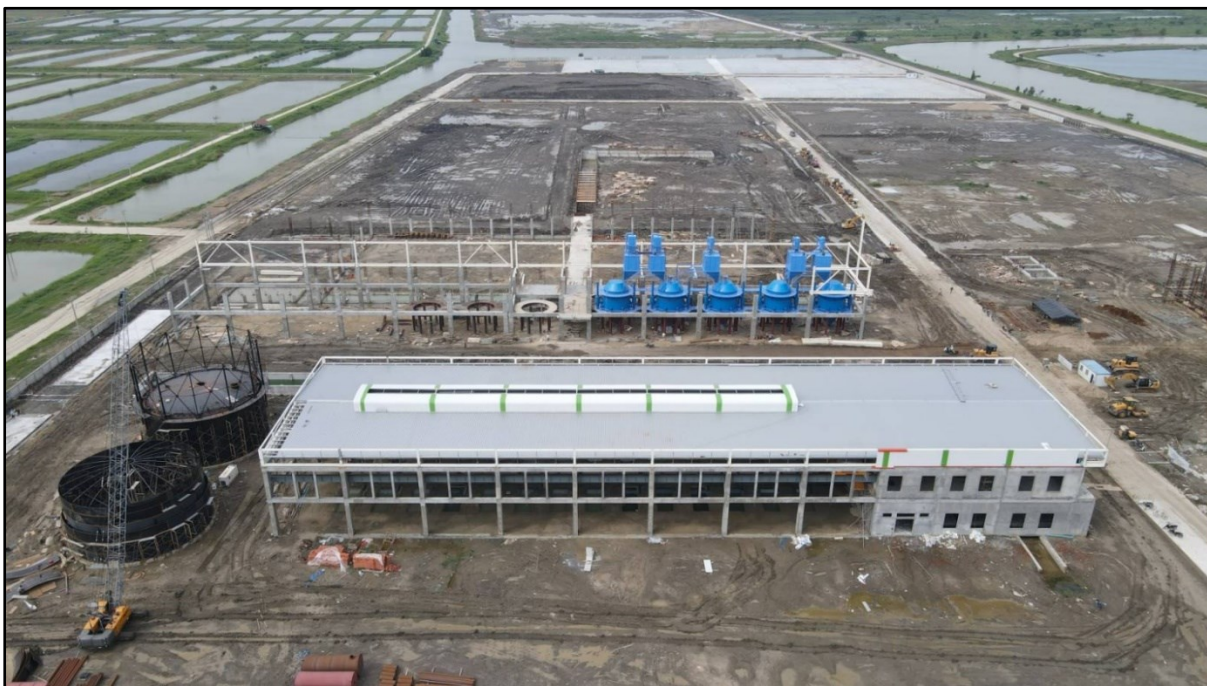
Photo (4.11) Biomass Power Plant
