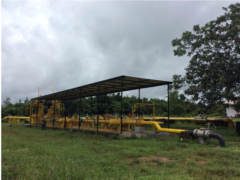
Figure 4. 14 Gas Metering Station
