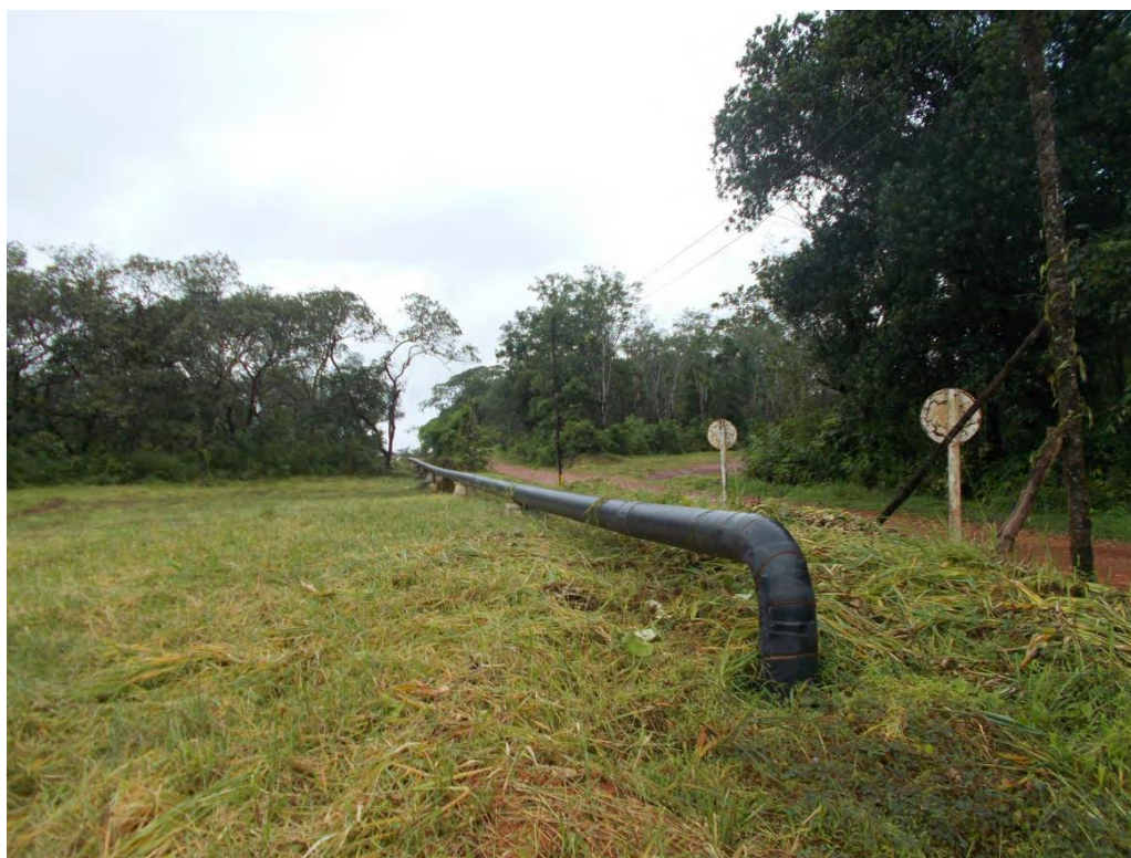
Figure 4. 16 Over Ground Portion of the Gas Pipeline
