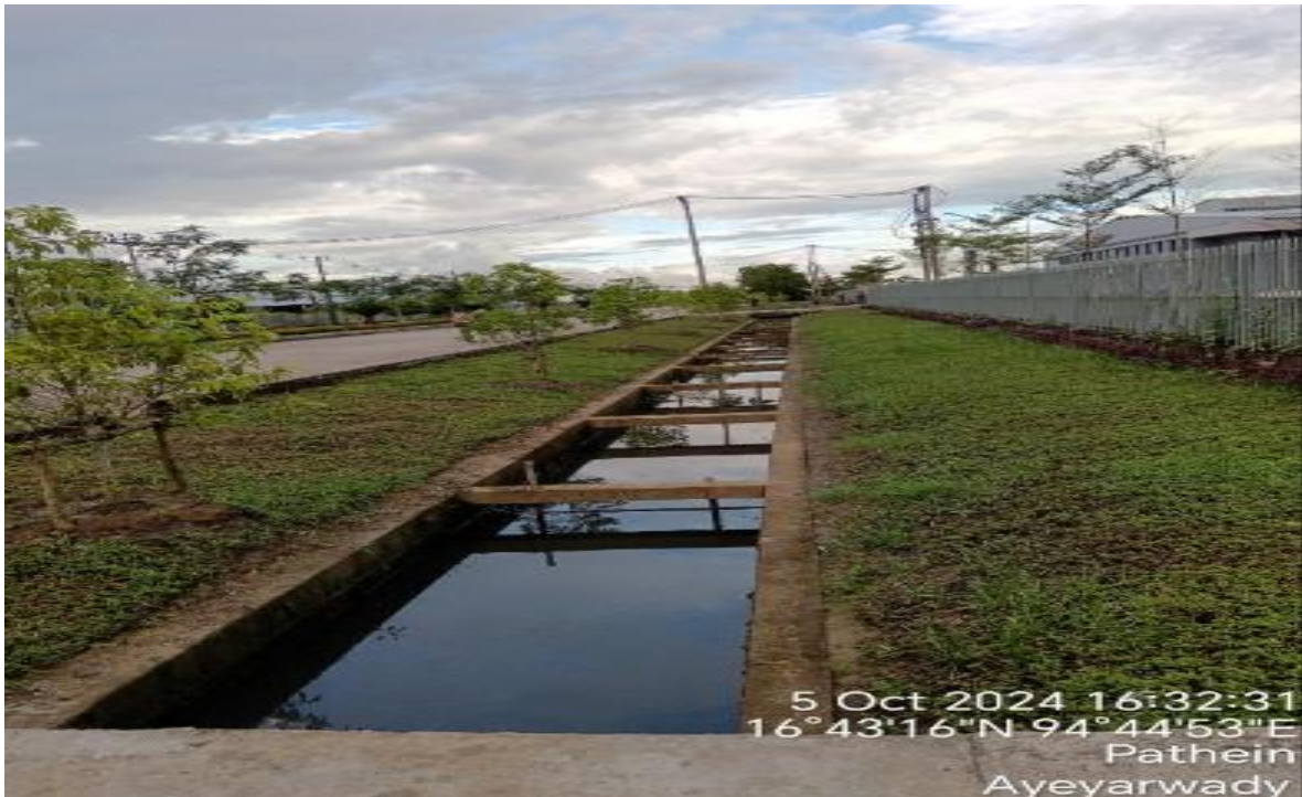
PIP Central Drainage
