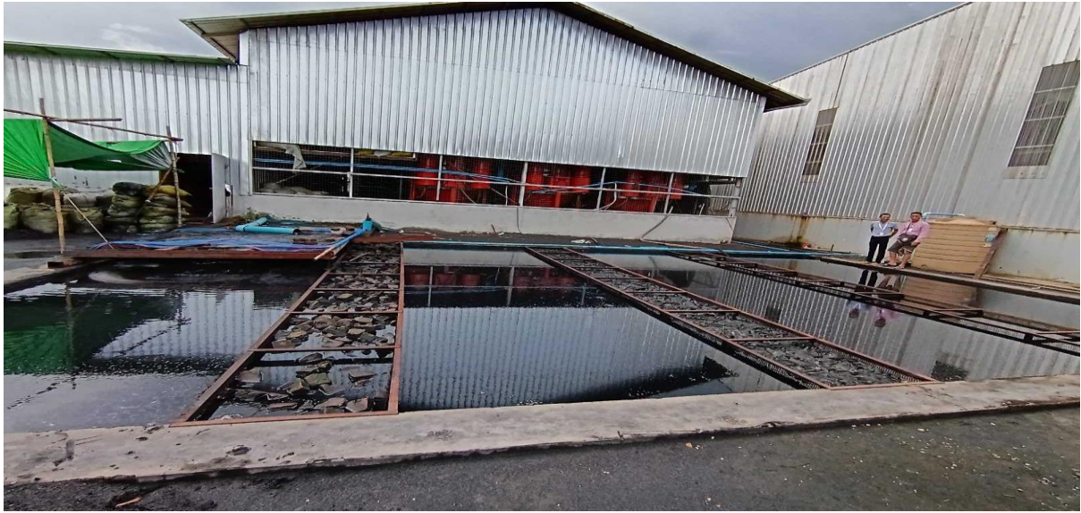
Figure 2-14 Wastewater Filtration Tank
