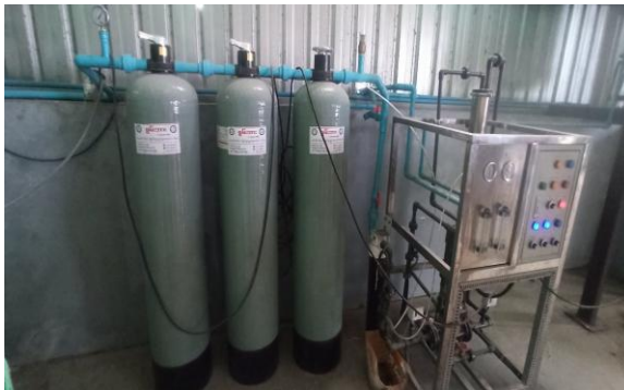
Water Purification System for Milling Operation
