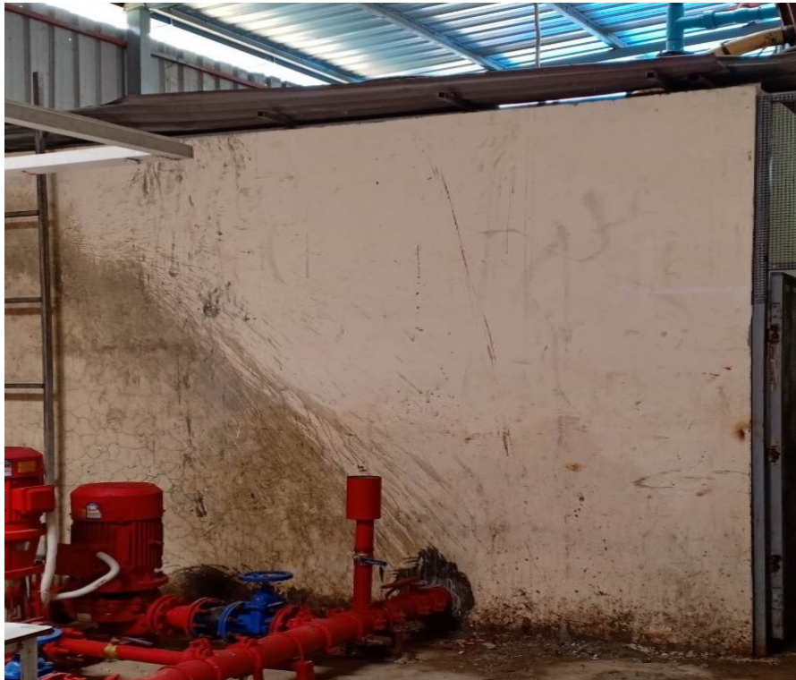
Figure 4-18: Photos of Water Supply
