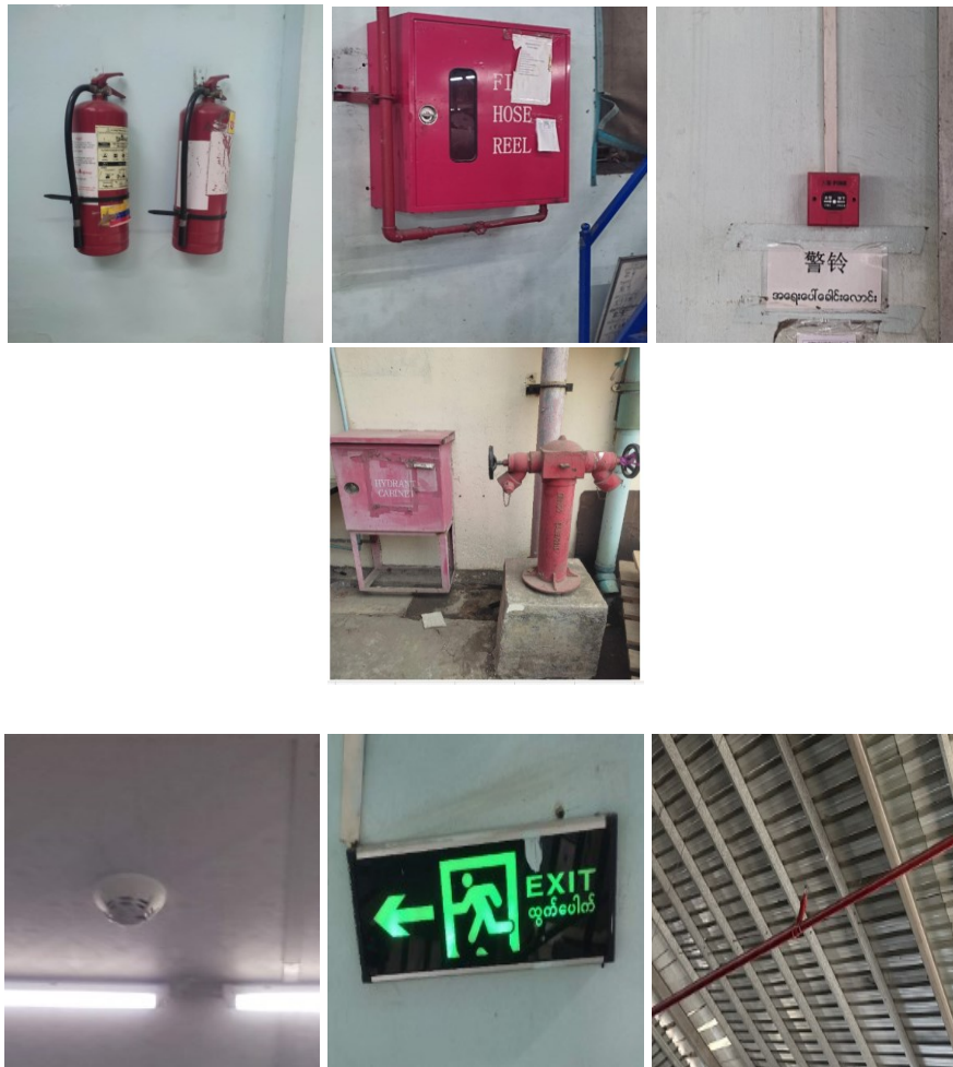
Figure 8-2: Photos of Facilities for Fire Prevention
