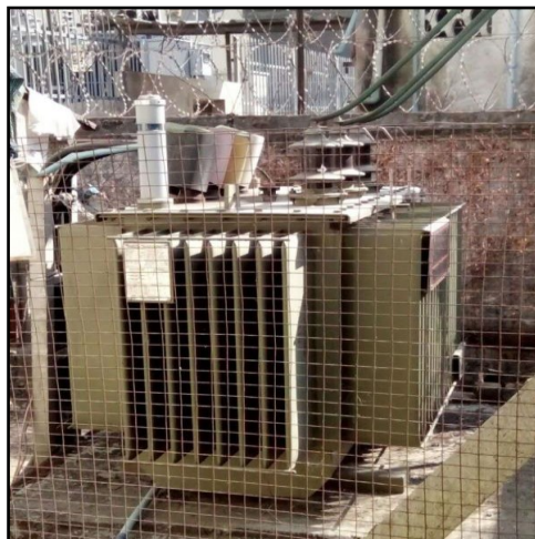
Figure 4-16: Photo of Transformer
