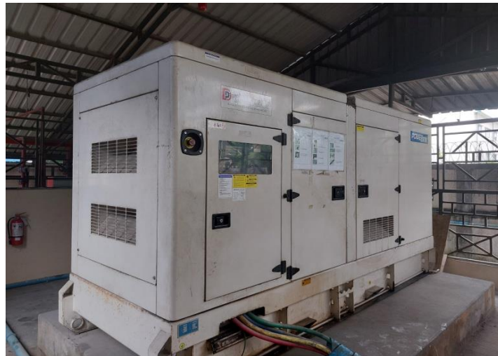
Figure 3-11 photograph of generator, 250 KVA
