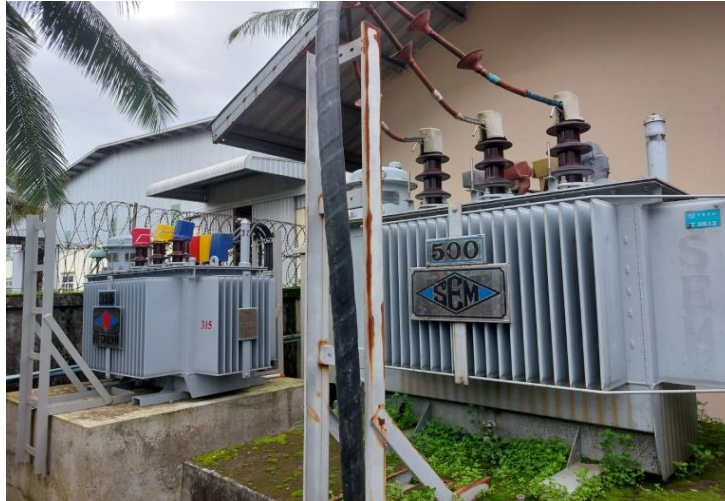
Figure 3-10 photograph of transformer; 537 H.P
