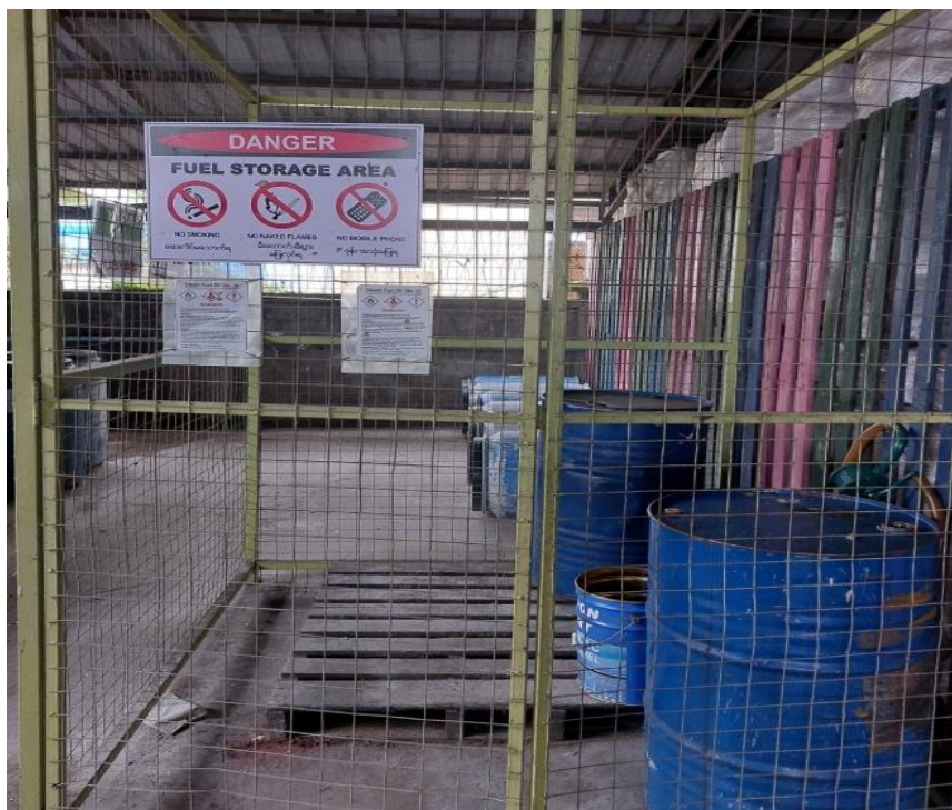
Figure 3-12 Diesel storage condition
