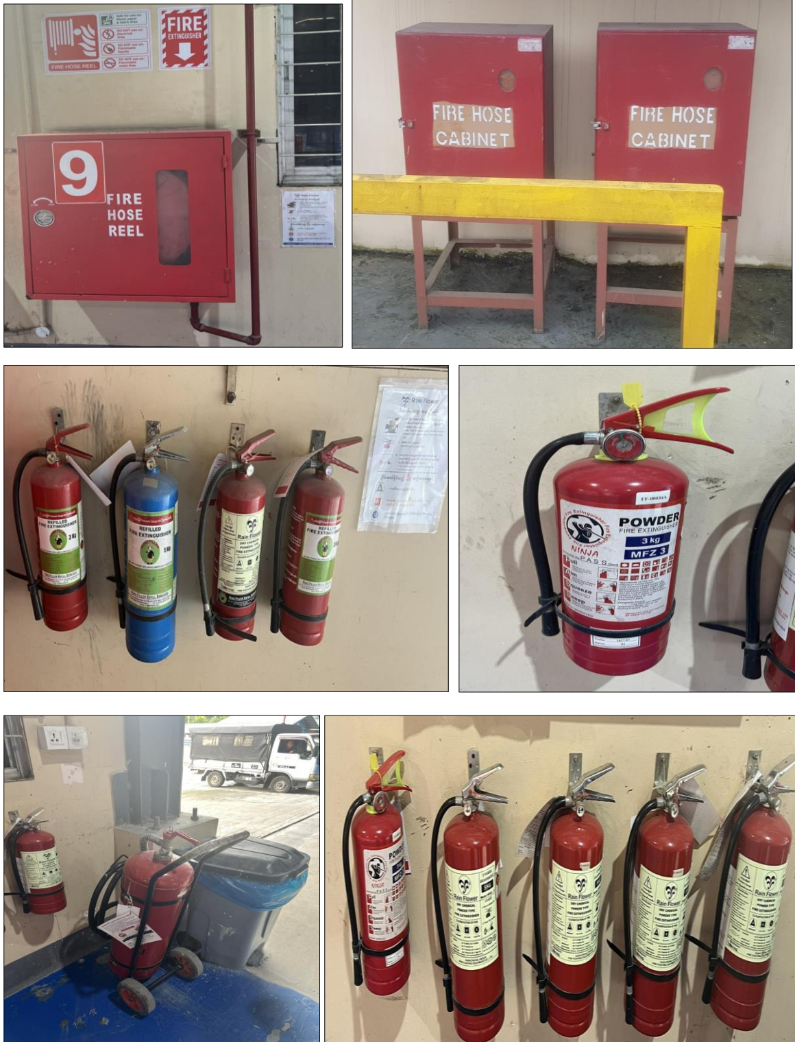
Figure 6-20 Fire Hose Reel and Fire Extinguishers
