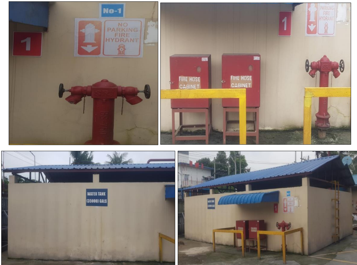
Figure 6-21 Fire Hydrants and Water Tank for Firefighting
