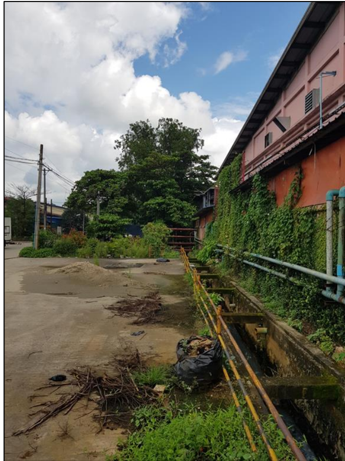
Figure 3.19: Wastewater Drainage Outside Factory
