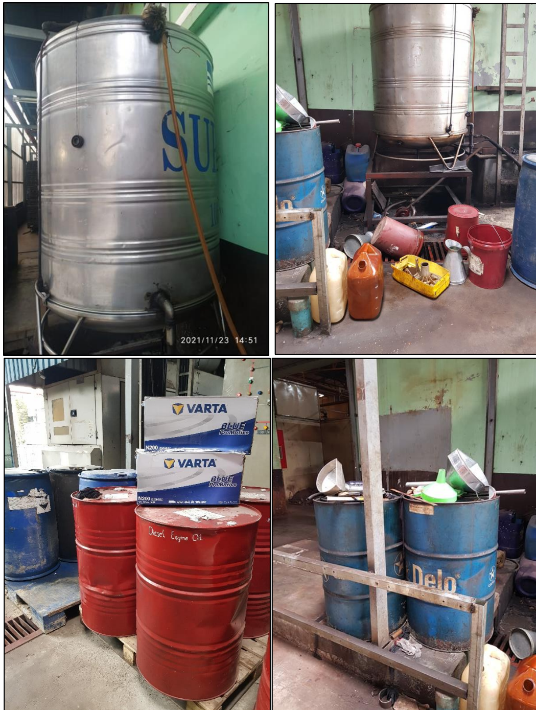
Figure 3.16: Fuel Storage near Generator
