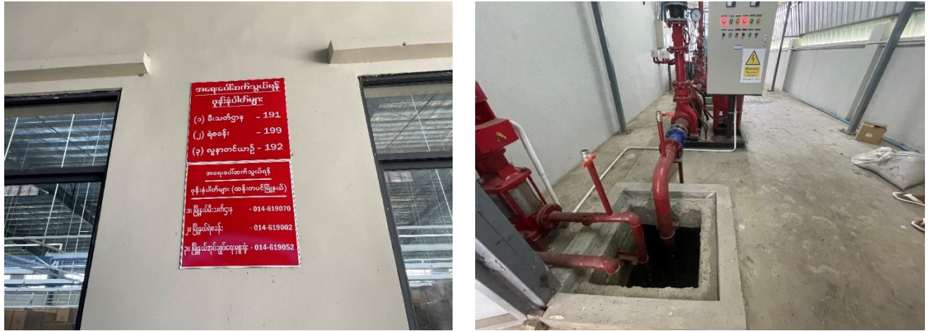
Figure 3.21 Emergency Safety and Fire Management System
