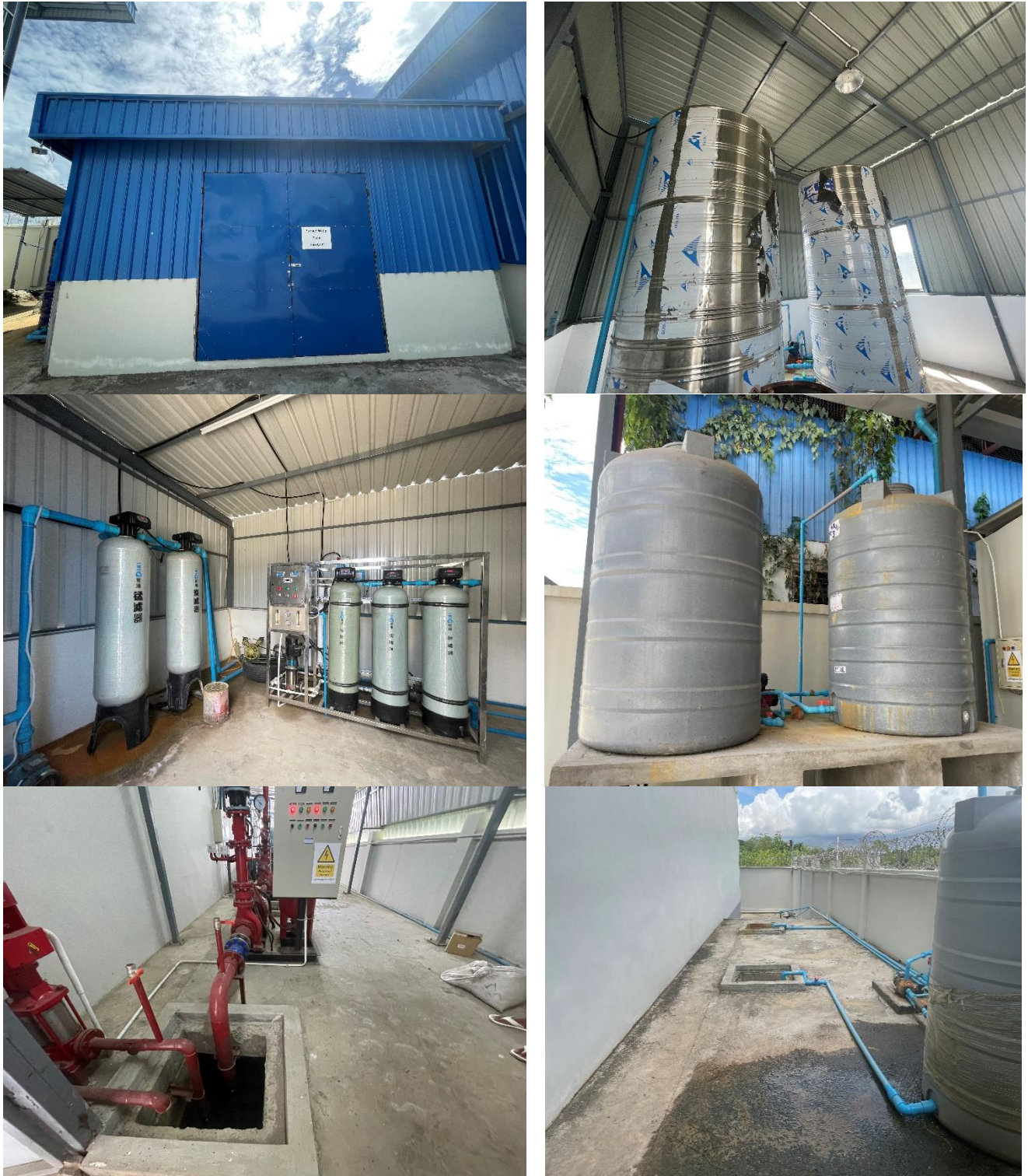
Figure 3.15 Water Storage Tank, Water Supply for Drinking Water and Firefighting
