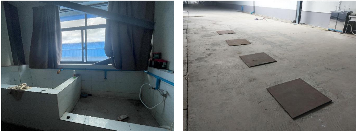
Figure 3.19 Used Mold Washing Area in Printing Department and Sedimentation Tank
