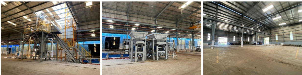
Figure 5-5 Condition of the Impermeable Floor Covering in The Factory
