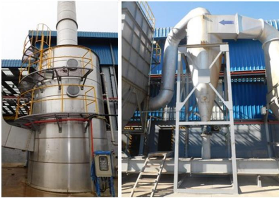
Figure 3-24 Exhausted (Dust & Gas) Setting & Cooling Chamber
