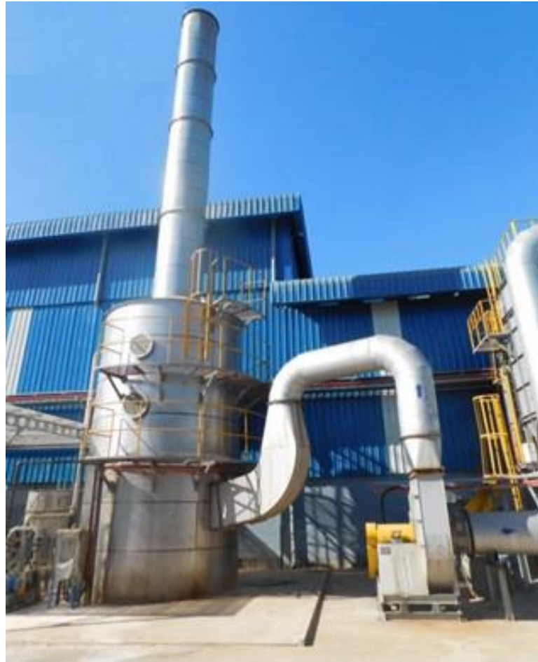
Figure 3-26 Blowing Fan and Wet Scrubber
