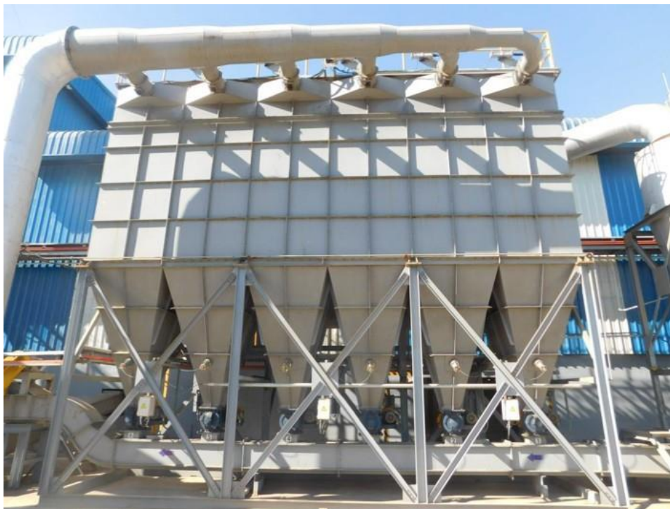
Figure 3-25 Filtering Bag House for Lead Dust of Rotary Smelter
