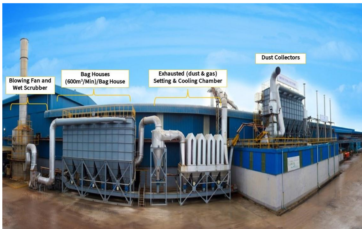
Figure 5-2 Air Emission Control Units in YMI Factory
