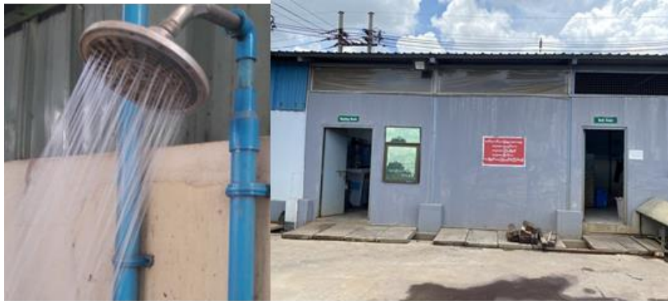
Figure 5-64 Sanitary Toilet, Bathroom, Closing Room and Eye Shower
