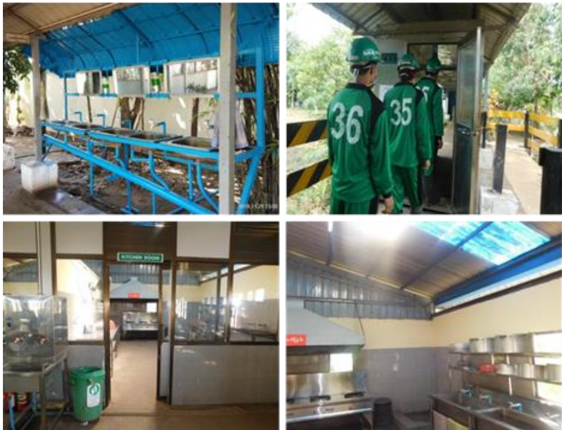
Figure 5-65 Air Blower Before Kitchen Room, Washing Facilities and Dining Room
