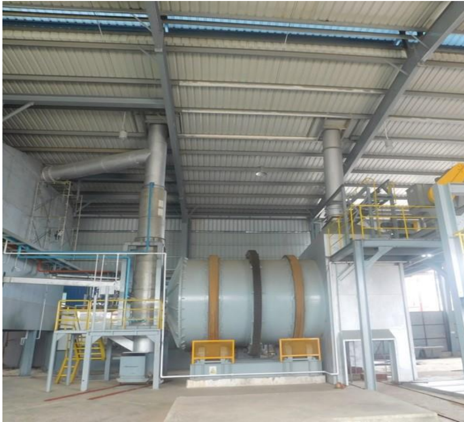
Figure 3-22 Rotary Furnace & Dust Line
