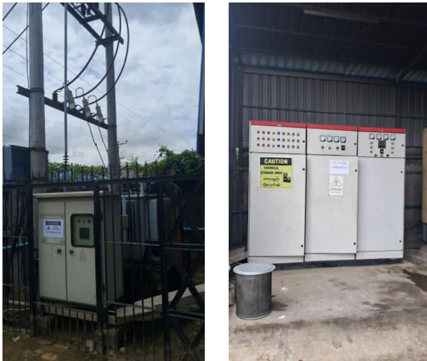
Figure 4-10 Power Transformer and Control Board
