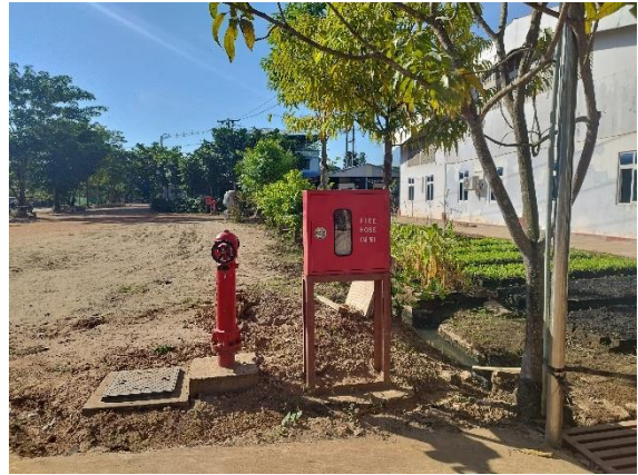
Fire Hose and Fire Hydrant
