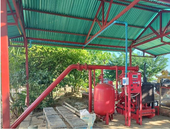
Fire Pump System
