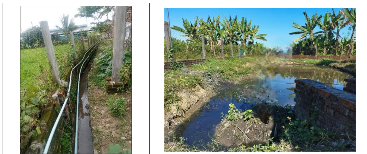
Figure 6.3 Drain and Natural Sedimentation Pond
