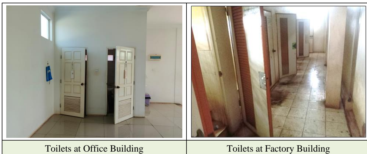
Figure 3.24 Photos of Septic Tanks and Toilets
