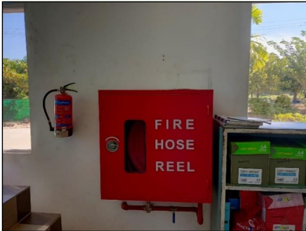
Fire Extinguisher and Fire Hose Reel
