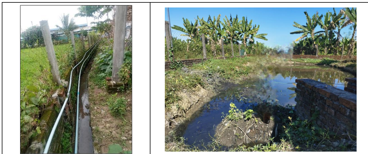
Figure 3.23 Drain and Natural Sedimentation Pond
